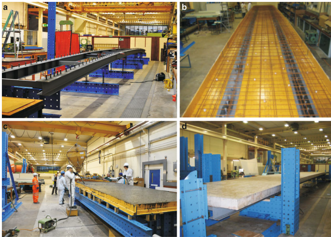
Fig. 41.2 Construction of the Warwick Bridge: (a) steelwork on six props, (b) preparation for casting, (c) casting of concrete and (d) final structure resting on two supporting frames
