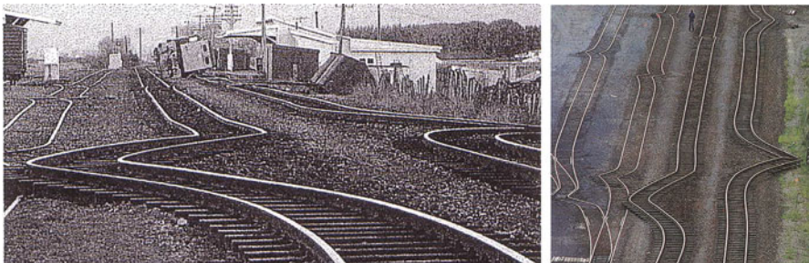
Fig. 8.6 The eastern Bay of Plenty (in New Zealand) was struck by a severe earthquake in March 1987. These photographs of Edgumbe railway station, with track bent in opposite directions, show the magnitude of the forces that were unleashed. (Left) – Ground level view, (right) – birds-eye view [26]
