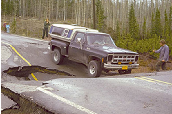
Fig. 13.4 Melting of permafrost causes a road to collapse in Alaska (Photo courtesy of Federal Highway Administration, 2010)
