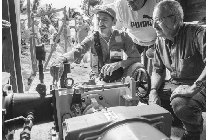
Micro-hydro plant near Santiago de Cuba.
