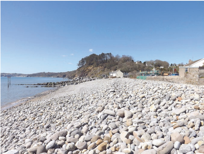
Fig. 3.11 Large cobbles added to the beach at Amroth, Pembrokeshire, to increase the stability of the beach and increase the protection from flooding of hinterland properties. © Greg Guthrie of Royal HaskoningDHV
