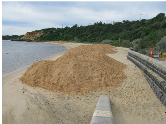
Fig. 4.1 Heaps of sand dumped on the beach at Half Moon Bay, Melbourne, Australia, prior to being spread on the renourished beach © Geostudies
