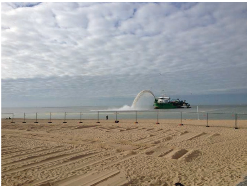
Fig. 4.13 Beach renourishment taking place at Ostend, Belgium in 2013. Sand extracted from the seafloor was pumping directly from the dredge barge to renourish the beach and nearshore areas. © Afdeling Kust
