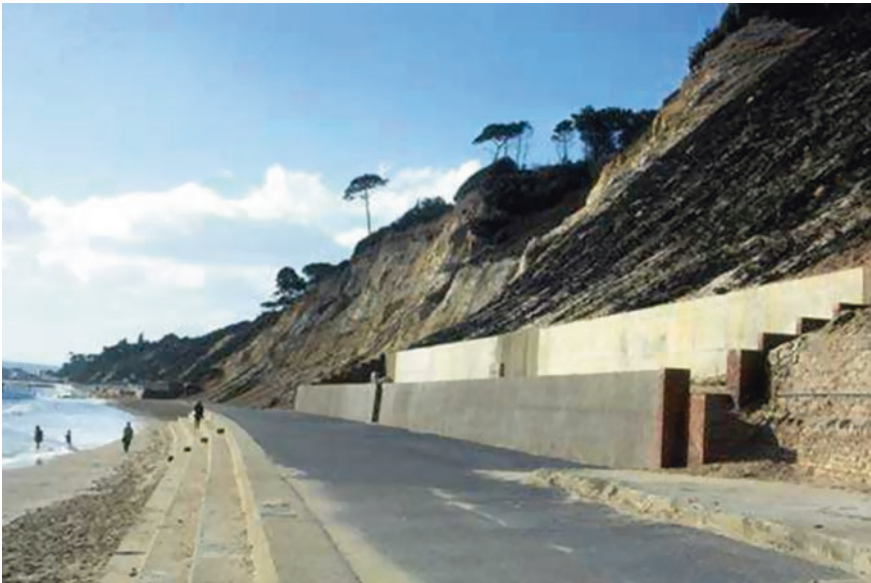
Fig. 2.4 Canford Cliff after the construction of a concrete esplanade along the base of the cliff. This halted marine erosion, but also reduced the supply of sand and gravel to adjacent beaches, which became depleted by marine erosion. © Geostudies
