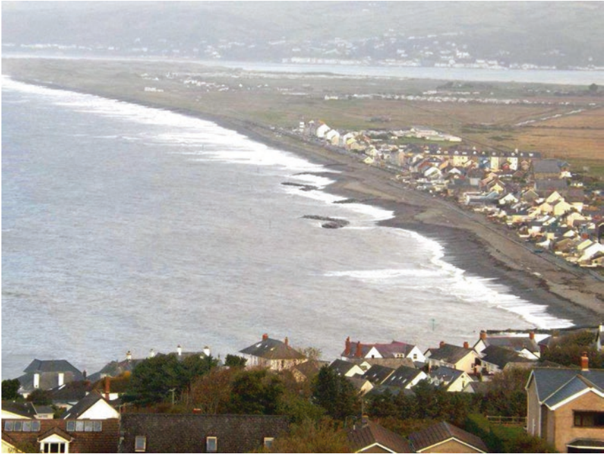
Fig. 3.7 Completed coastal protection works at Borth, United Kingdom. Beach renourishment supplemented a submerged rock berm and two breakwaters. © Royal HaskoningDHV
