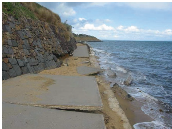
Fig. 3.1 Storm-damaged sea wall at Black Rock, Victoria, Australia. © Geostudies
