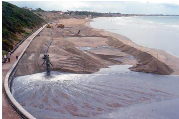
Fig. 4.12 Sand pumped on to the shore at Mentone, Port Phillip Bay, Australia, and deposited as a renourished beach. © Geostudies
