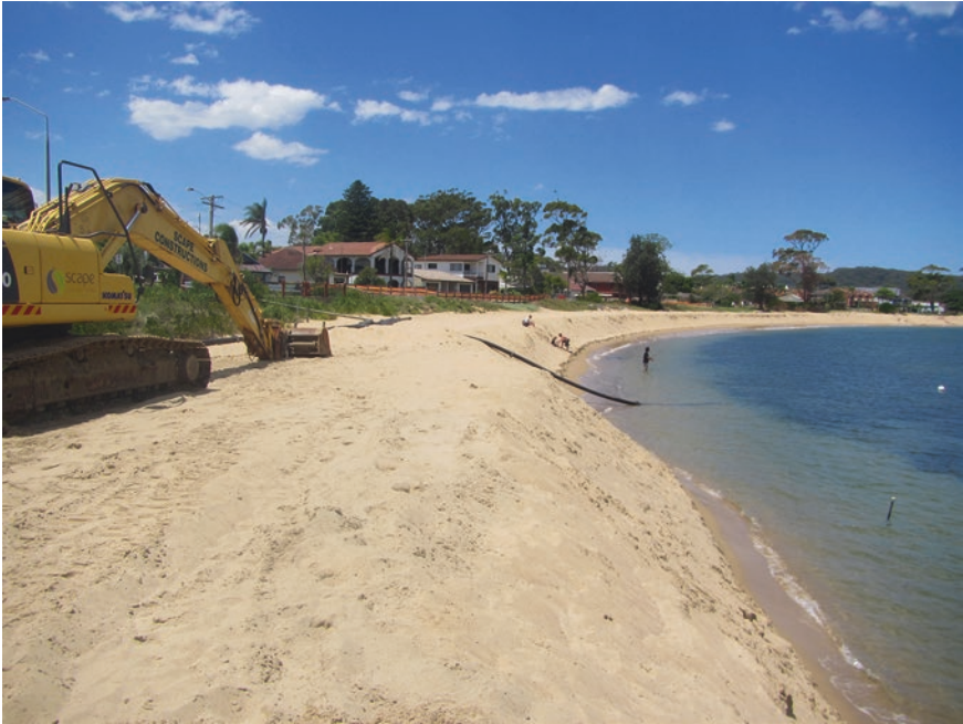
Fig. 6.2 Renourishment of Ettalong Beach, Broken Bay, Australia during November 2013. Sediment dredged from the bay floor 1 km offshore is pumped onshore through a hydraulic pipe and then placed in heaps along the sub-aerial beach by excavator. © Nick Lewis
