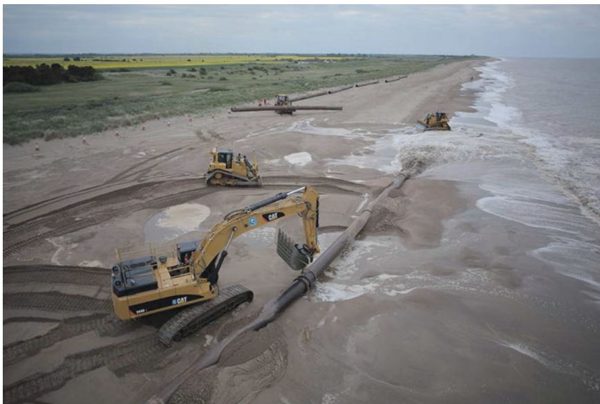
Fig. 6.1 Beach renourishment on the Lincolnshire coast, United Kingdom. Between 2010 and 2015 15,000 m 3 of sediment per day was pumped ashore and placed on the beach using hydraulic pipes. Sediment was then spread across the beach using excavators and bulldozers. © Dredging International
