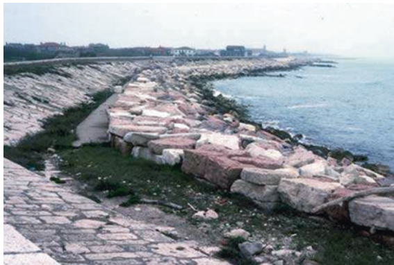
Fig. 3.10 After a sea wall and groyne failed to retain a beach at Litorale di Palestrina on the NE coast of Italy limestone boulders were dumped on the shore. © Geostudies
