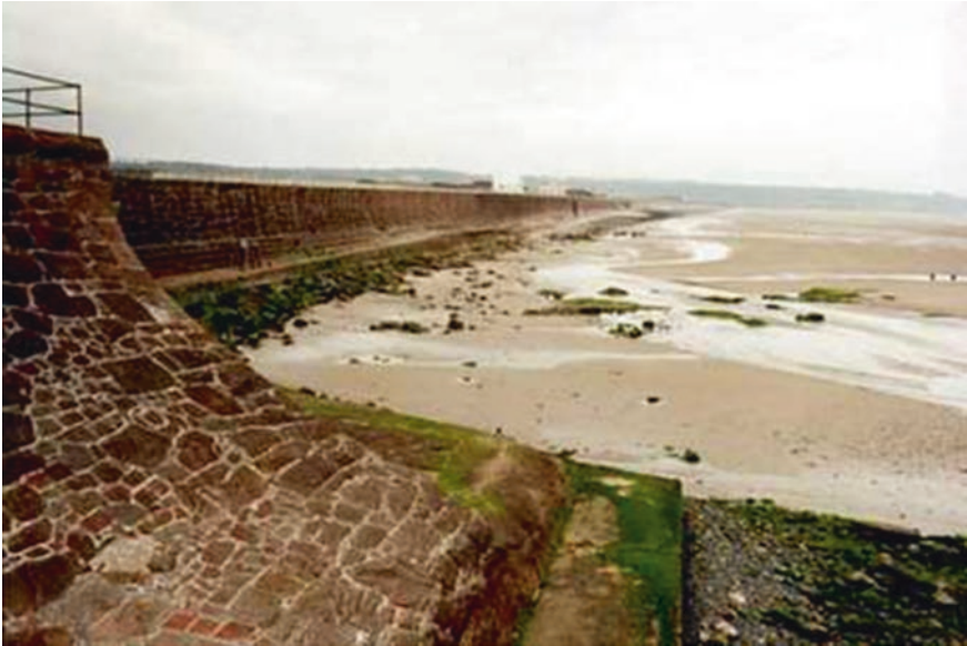
Fig. 2.18 The sea wall at St Ouen's Bay, Jersey, with the beach lowered by reflection scour. © Geostudies
