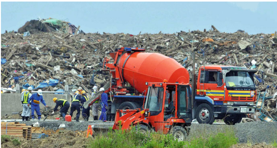
Fig. 1.48 Concentrated mix debris in Kesenuma City awaiting for recycling
