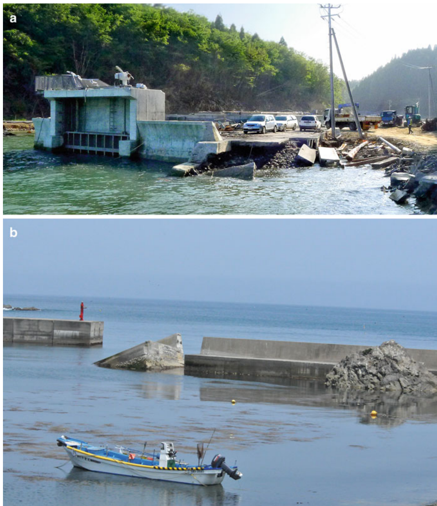
Fig. 1.43 (a) and (b) Sluice gate ( above ) and seawall ( below ) overpowered by the tsunami along the Sanriku coastline
