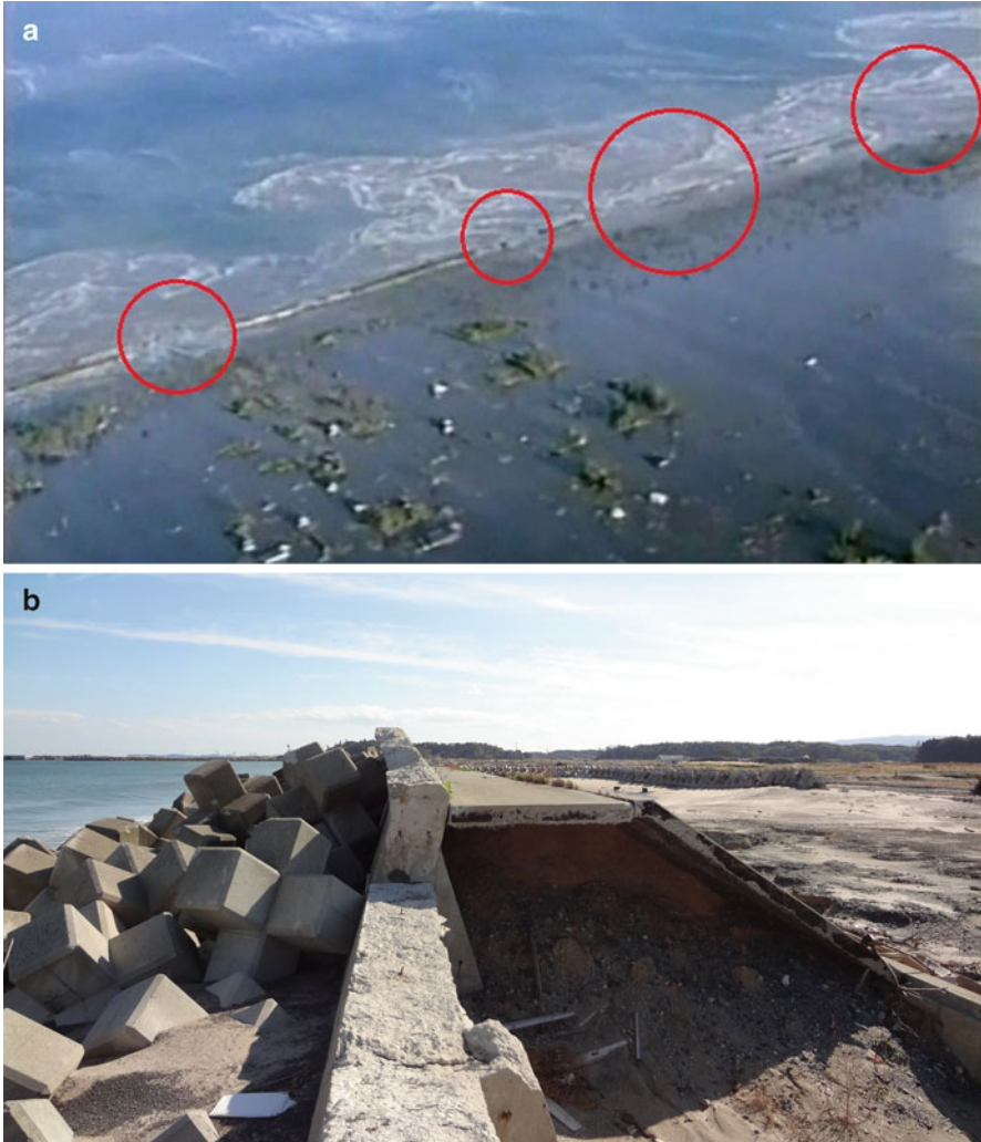
Fig. 16.8 (a) JLT 16:39 Breaking of the upper structures on the Yamamoto Coast taken by “Michinokugo”. (b) Breaking of the upper structure on the Yamamoto Coast
