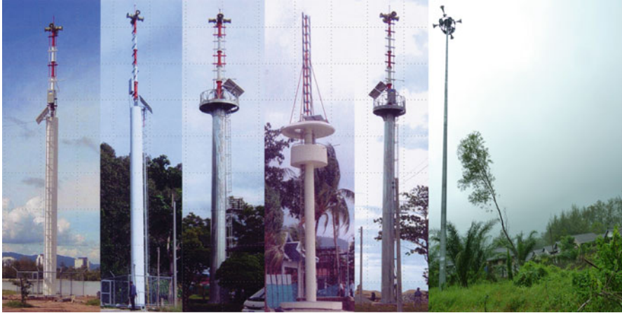
Fig. 23.4 Various types of the warning towers operated by the NDWC ( left ) and a warning tower built by the local government at Ban Suk Samran, Ranong province ( right : photo taken in August 2012)
