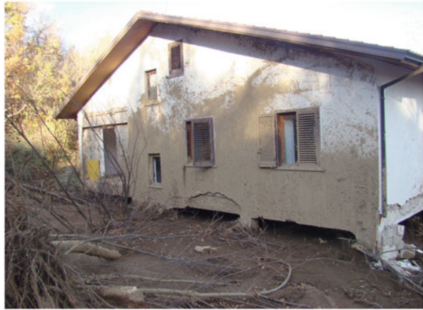
Fig. 13.4 Photo of the southern side of the house involved by the debris avalanche
