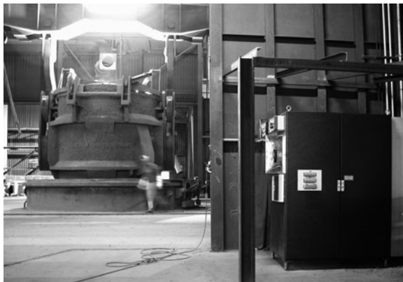
Fig. 18.6 LIBS instrument installed in a steel plant (in front on the right)
