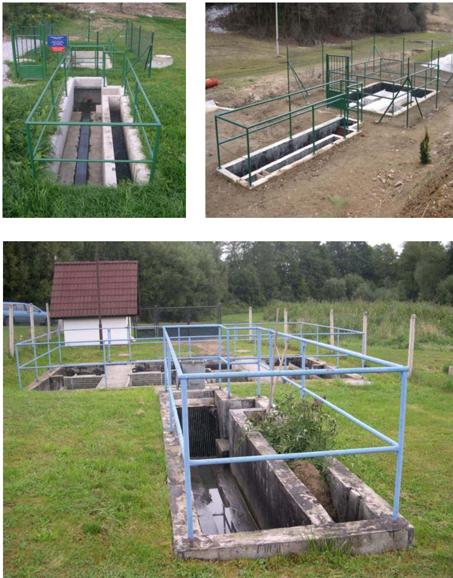
Figure 5-15. Examples of pretreatment for secondary treatment HF constructed wetlands for 100 PE (top left, Petrovice, Czech Republic), 200 PE (top right, Skuhrov, Czech Republic) and 500 PE (bottom, Dolní Město, Czech Republic). All systems consist of screens, horizontal grit chamber and Imhoff tank. Photos by Lenka Kröpfelová.
