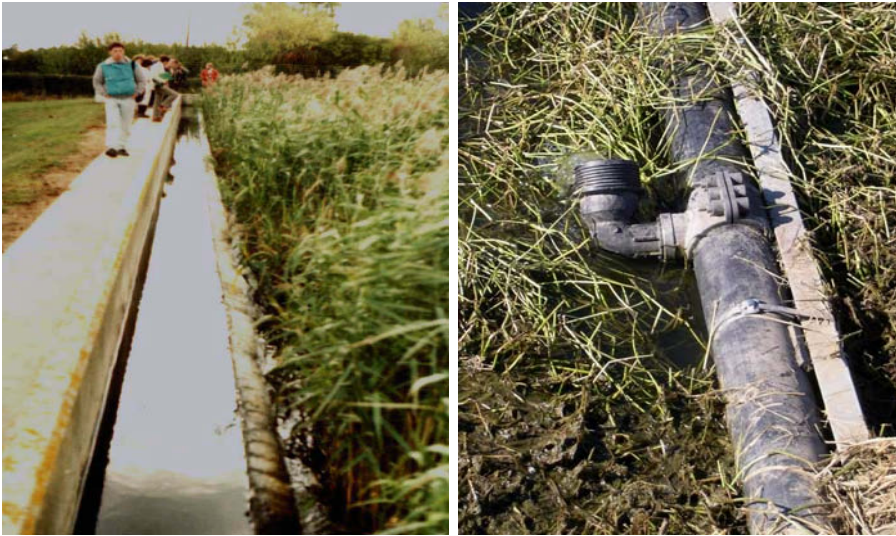
Figure 5-24. Open inflow trench in HF CW Acle, United Kingdom (left) and adjustable tees in HF CW Otorohanga, New Zealand (right). Photos by Jan Vymazal.
