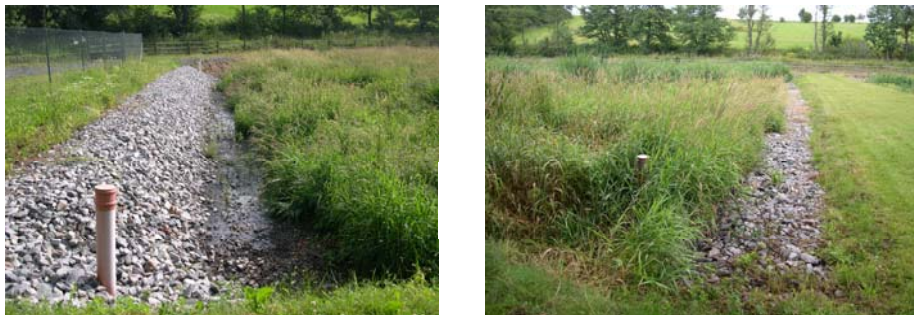
Figure 5-17. Inflow and outflow zones in CW Obecnice, Czech Republic. Photos by Lenka Kröpfelová.
