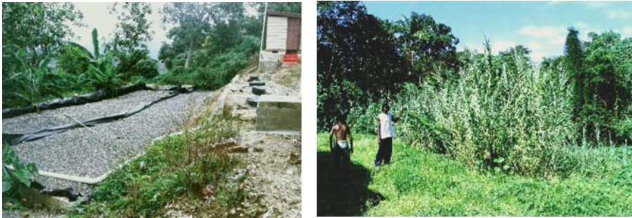
Figure 7-43. HF constructed wetlands at Pigsaw (left, before planting) and Retrieve (right, planted with wild cane, Gynerium sagittatum ) in Jamaica. Photos by Ed Stewart, with permission.
