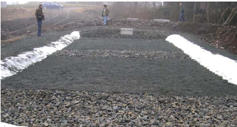
Figure 7-22. HF constructed wetland for secondary treatment of municipal sewage at Zadný Hámor, East Slovakia (17 PE, 90 m 2 ) after completion in November 2006. Photo by Jan Vymazal.
