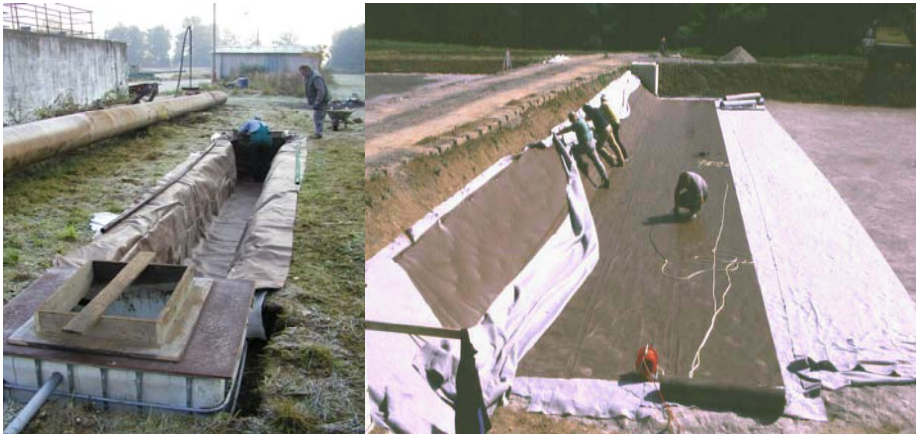
Figure 5-16. Left: plastic liner at the experimental HF constructed wetland at Třeboň, Czech Republic. Right: Plastic liner in between two layers of geotextile (CW Mořina, Czech Republic). Photos by Jan Vymazal.
