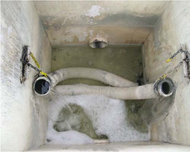
Figure 5-35. Flexible hoses at the outflow from a HF CW Mořina, Czech Republic. Photo by Jan Vymazal.
