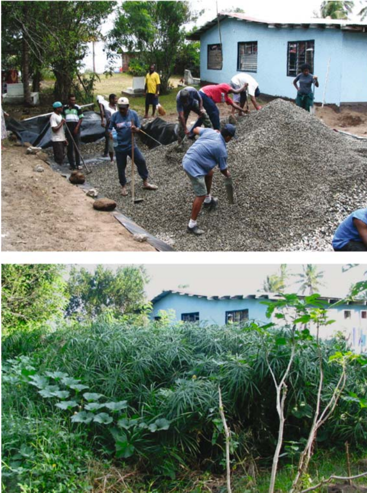
Figure 7-50. HF constructed wetland at Tangage, Fiji planted with Cyperus involucratus . Photos by Chris Tanner, with permission.
