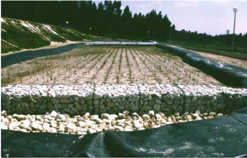
Figure 6-9. HF constructed wetland as a part of a VF-HF hybrid constructed wetlands for landfill leachate in Leiria, Portugal. Photo by Jan Vymazal.
