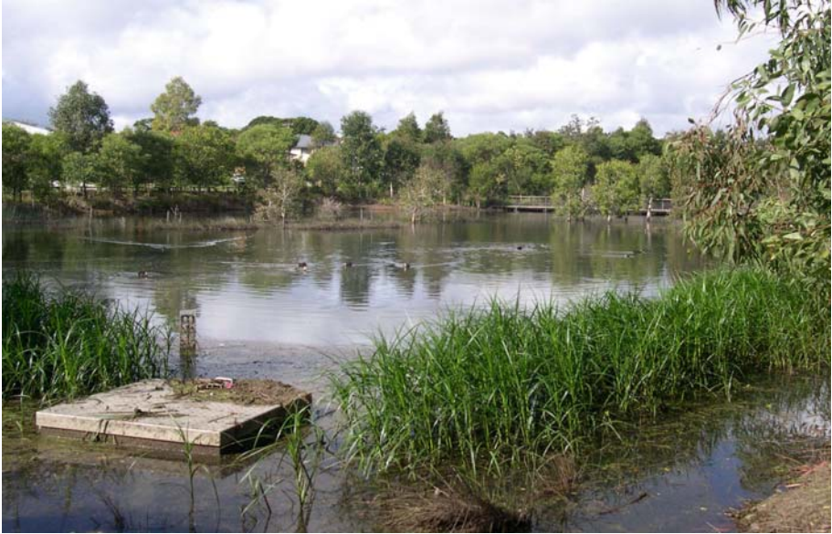
Figure 4-20. Outflow structure in a stormwater treatment constructed wetland, Brisbane, NSW, Australia. Photo by Jan Vymazal.
