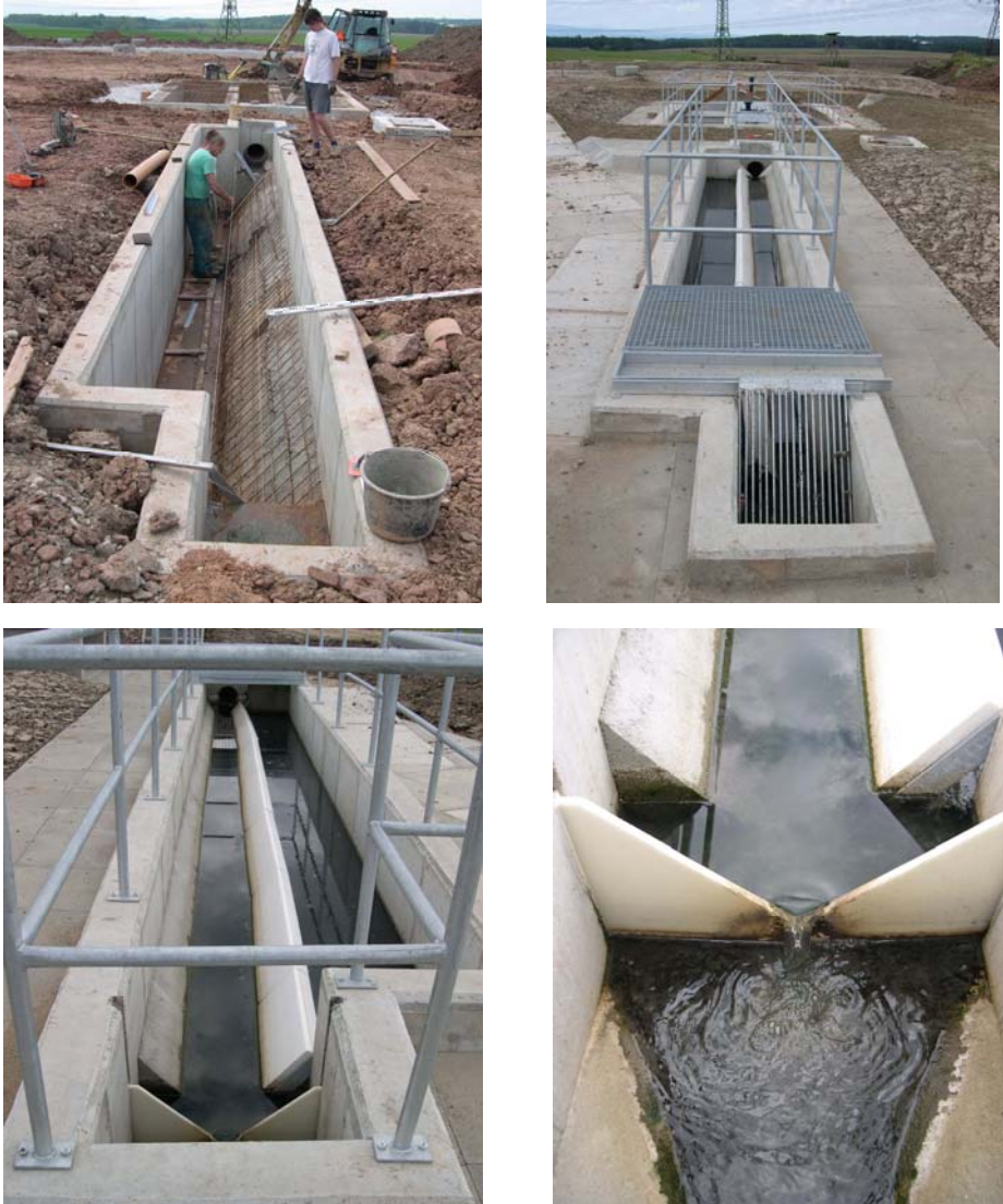
Figure. 5-12. Horizontal flow grit removal chamber in CW Libnič, Czech Republic. Top left: during the construction, note the depth of a sludge compartment, top right: grit chamber with screen bars after completion, bottom left: the view from the outflow side with the triangle trough in the left, bottom right: detail of the weir. Photos by Lenka Kröpfelová.
