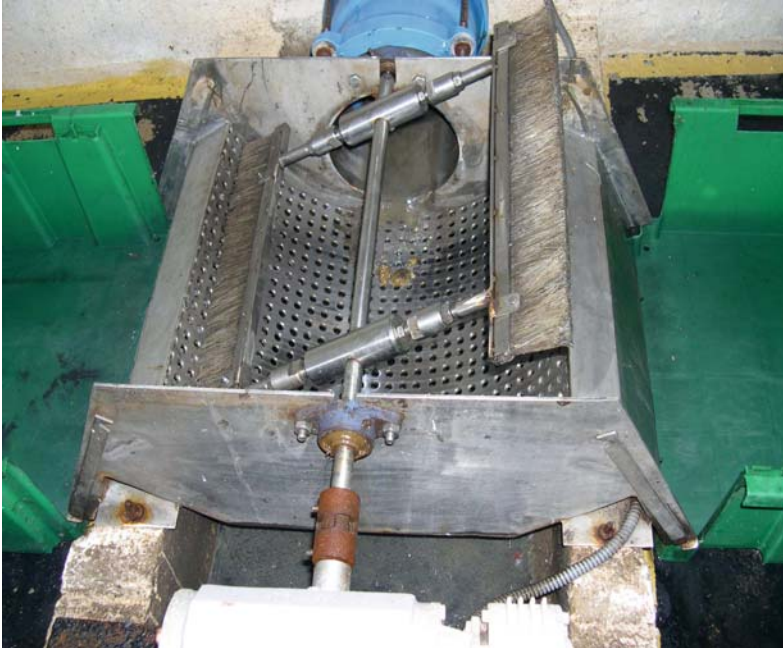
Figure 5-9. Mechanically-cleaned screens at constructed wetland Beja, Portugal. Photo by Lenka Kröpfelová.
