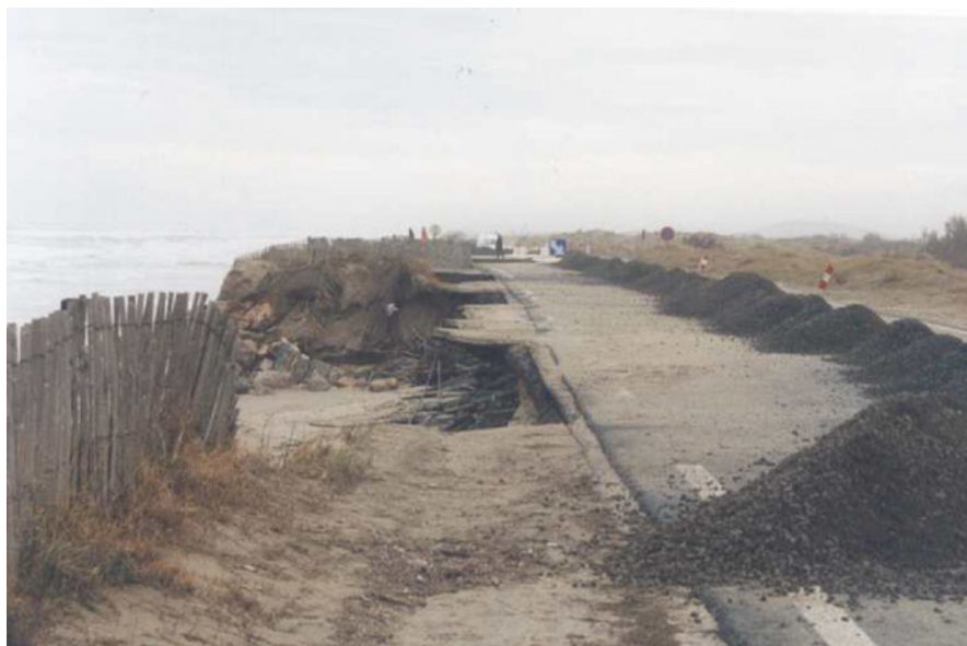
Fig. 4.19 Recurrent erosion impacts on the coastal road
