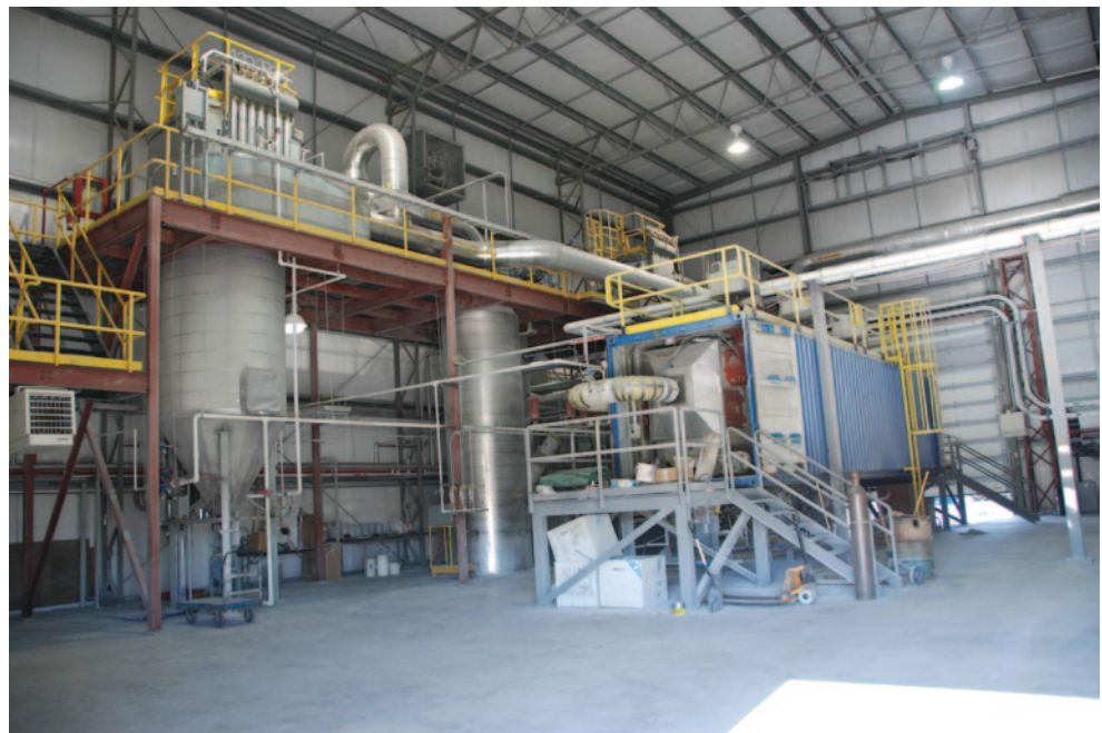
Fig. 9.4 Enhanced electrostatic precipitator at poplar river power station near Coronach, Saskatchewan. (Photo provided by and property of SaskPower)
