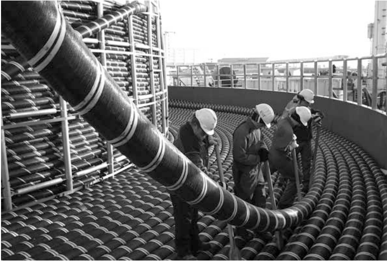
Figure 8.1 At 580 km the NorNed link between Kvinesdal, Norway, and Eemshaven, the Netherlands, is the world's longest high-voltage submarine power cable. Here the cable is loaded onto the cable-laying vessel.
