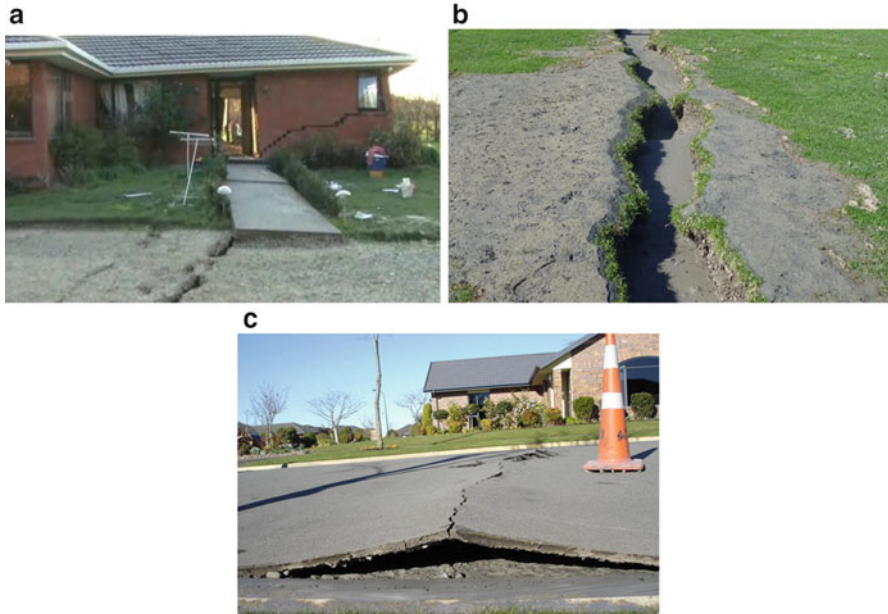
Fig. 4.66 Damage to house, ground fissure and buckling of pavement (2010 Darfield earthquake, New Zealand). (a) A House damaged by ground displacement. (b) Ground fissure and sand boil. (c) Buckling of pavement
