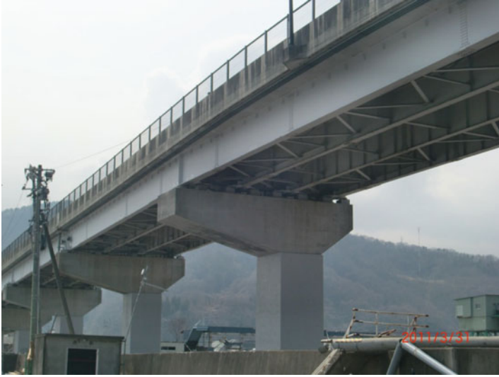
Fig. 1.96 A concrete viaduct for road survived from the tsunami (2011 Tohoku earthquake, at Kamaishi)
