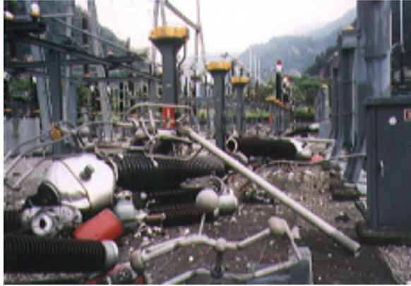
Fig. 1.20 Collapse of air circuit breakers by strong ground motion and earthquake fault offset (1999 Chi-Chi earthquake, Taiwan)
