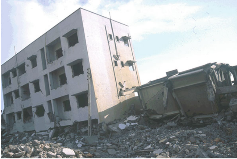
Fig. 1.27 Collapse of Piloti-type concrete building (2001 Gujarat-Kachchh earthquake, India, at Ahmadabad)
