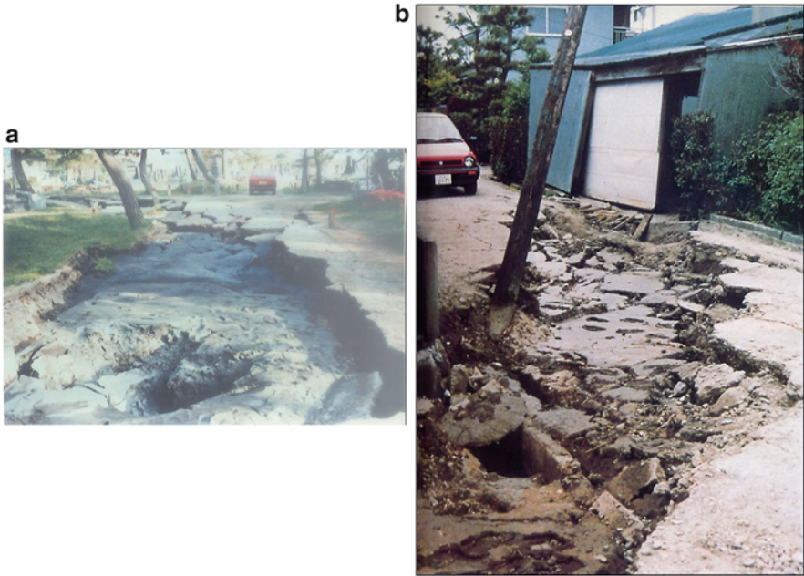
Fig. 4.2 Surface fissures by horizontal ground displacements (1983 Central Japan Sea earthquake). (a) Surface fissure and sand volcano in a park. (b) Surface fissure in a residential area
