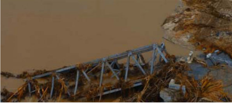
Fig. 1.37 Steel truss bridge washed down by the tsunami (2004 Sumatra offshore earthquake and tsunami, on the west coast of Sumatra)
