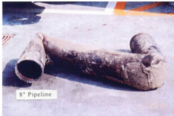
Fig. 1.19 Buckling of a gas pipe by earthquake fault offset (1999 Chi-Chi earthquake, Taiwan)
