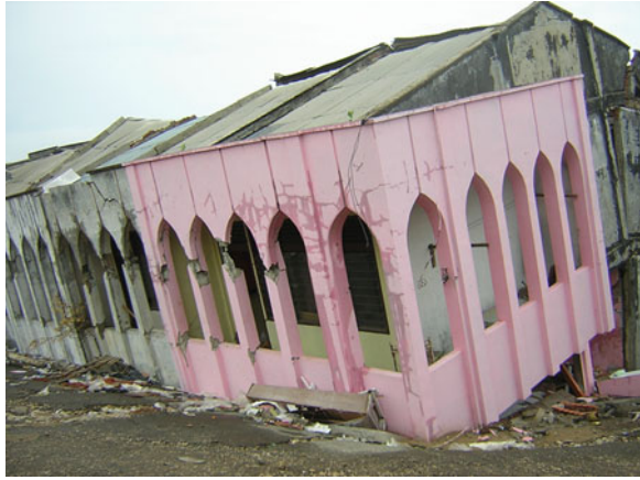
Fig. 6.31 Subsided and Inclined building due to soil liquefaction (2005 Nias Island earthquake, Indonesia)
