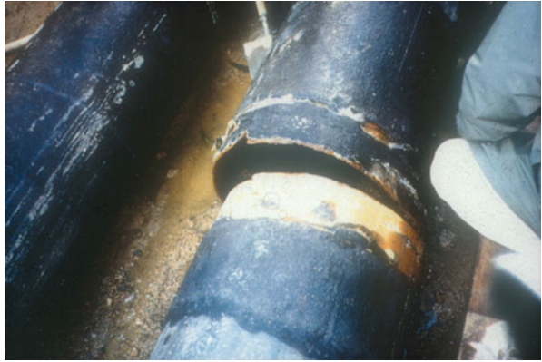
Fig. 4.40 Rupture of buried pipe of water trunk line by liquefaction-induced ground displacements (1995 Kobe earthquake, Port Island)
