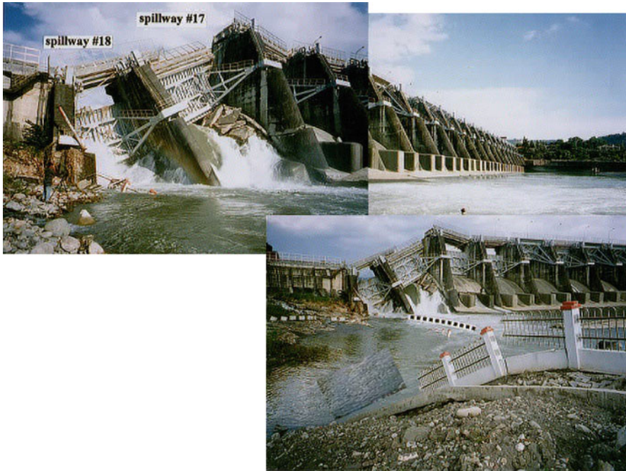
Fig. 1.15 Destruction of Shin-Kang dam caused by the earthquake fault (1999 Chi-Chi earthquake, Taiwan)
