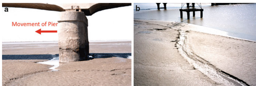
Fig. 1.26 Movement of bridge pier due to liquefied ground displacement (2001 Gujarat-Kachchh earthquake, India, at Hadakia bridge). (a) Movement of pier. (b) Soil liquefaction and surface break
