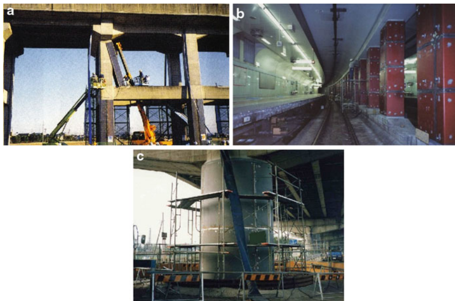
Fig. 2.24 Seismic reinforcement of concrete structures (by steel jacking). (a) Concrete viaduct of shinkansen ( new trunk line ). (b) Center concrete column of subway station. (c) Concrete bridge pier of an express way
