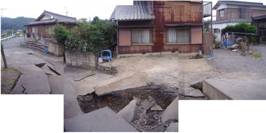
Fig. 6.16 Cave-in due to collapse of lignite mine
