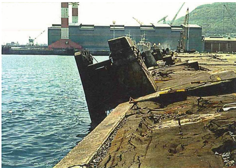
Fig. 1.54 Deformation and inclination of quay wall by steel sheet piles at Hakodate port (1993 Southwest Hokkaido offshore earthquake)
