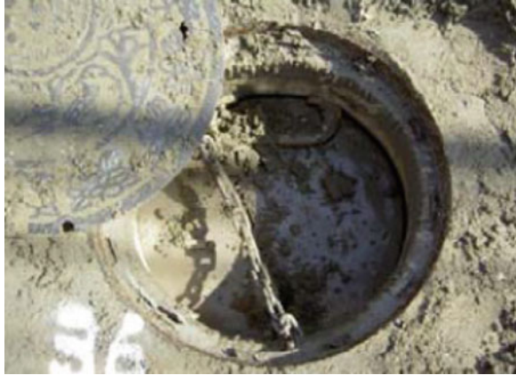
Fig. 2.9 Liquefied soil flow into a manhole (2011 Tohoku earthquake)
