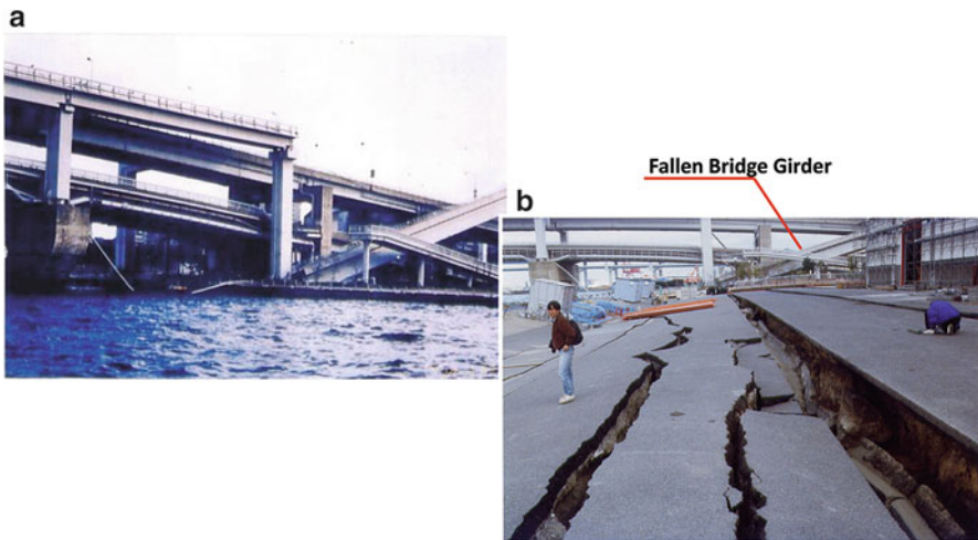
Fig. 4.35 Fall of a bridge girder by liquefaction-induced ground displacements (1995 Kobe earthquake, at Rokko Island). (a) Fall of a bridge girder. (b) Ground fissures, and inclination and subsidence of ground surface
