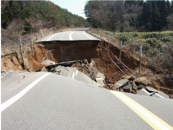
Fig. 1.81 Failure of embankment of a highway crossing vally (2007 Noto Peninsula earthquake)
