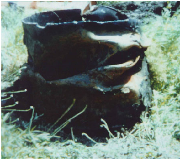
Fig. 1.9 Buckling of buried pipe due to earthquake fault offset (1999 Kocaeli earthquake, Turkey, at Arifiye)
