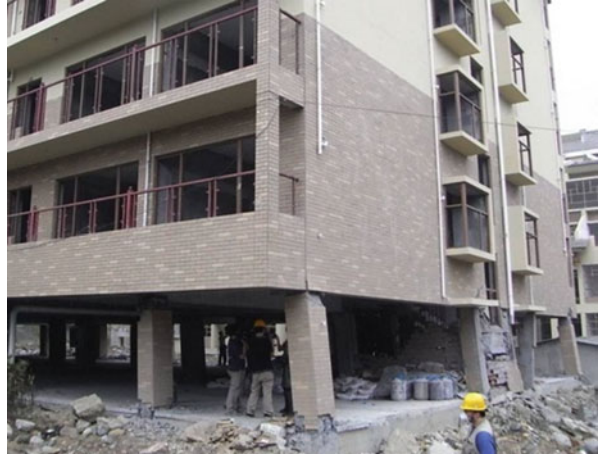
Fig. 6.33 Damage to reinforced concrete building (2008 Wenchuan earthquake in Shichuan province, China)
