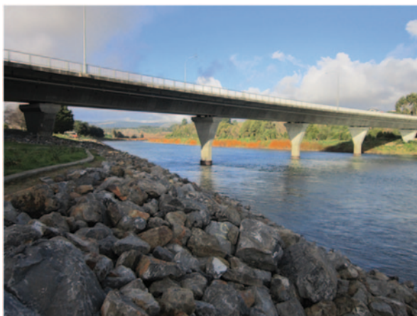
Fig. 10.5 Stopbanks and rock revetments, Fitzherbert Bridge, Palmerston North. (Source: Bruce C. Glavovic)
