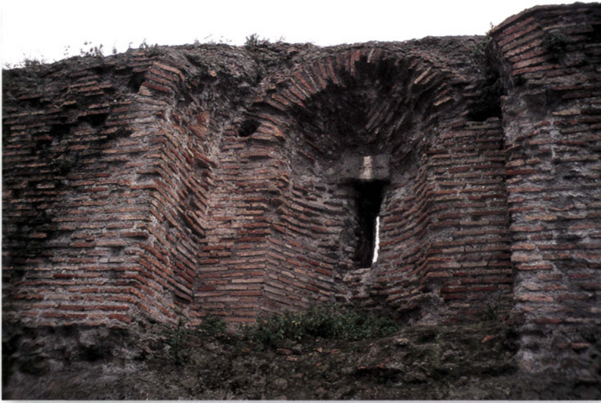
The brick-faced concrete construction on the interior of a tower in Viale Giotte. Once properly set, it created a homogeneous mass that was less vulnerable to collapse than dry stone construction. (Author's collection)
