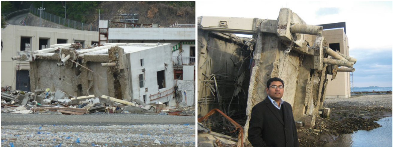
Fig. 2 Pile building failure in Onagawa during 2011 Japan earthquake
