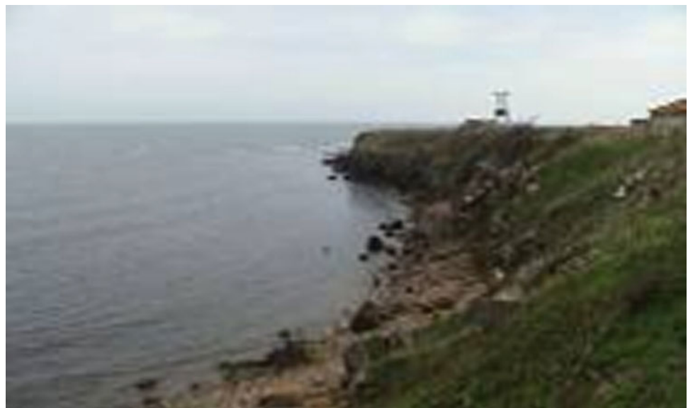
Fig. 8 Section of the north coast of Primorsko affected by landslides and rock falls before the construction of retaining structures
