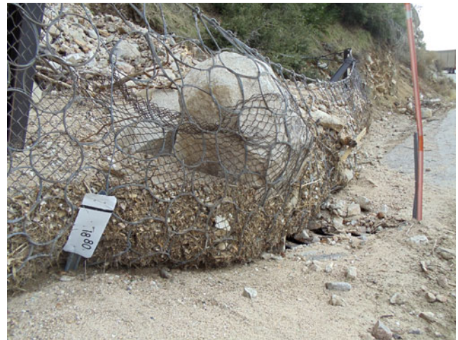
Fig. 8 Site 7 December 2010 debris (Courtesy Duffy)
