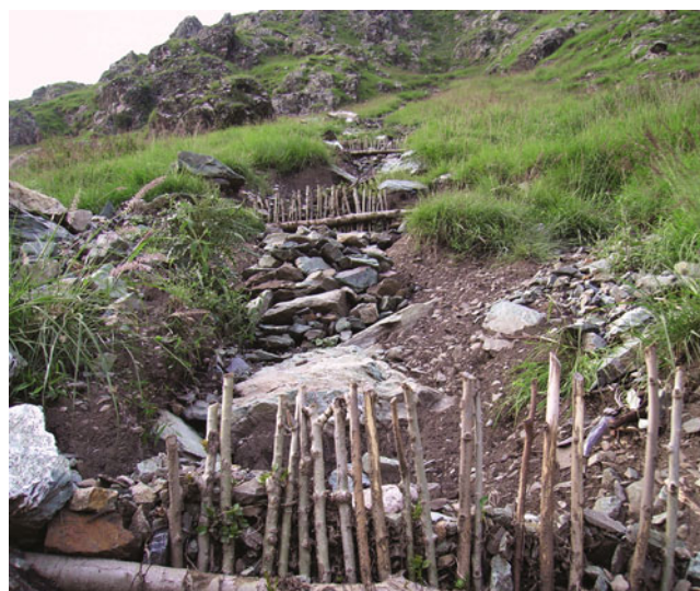
Fig. 3 Palisade – a successful bio-engineering technique for landslide stabilization introduced and field-tested by the project (Photographer: Paolo Ceci, FAO)
