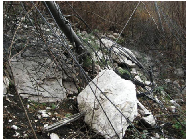
Fig. 12 Crashed barrier after rockfall event
