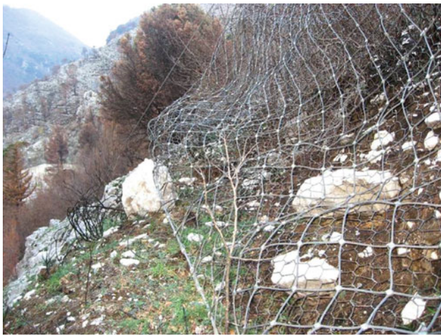
Fig. 11 Boulders passing underneath old-concept rockfall barrier
