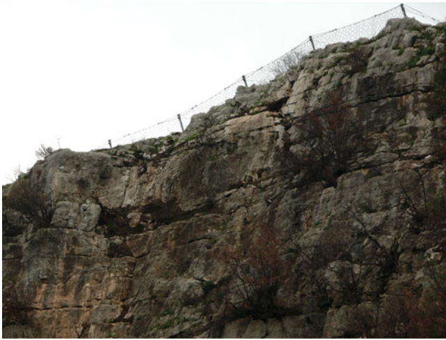
Fig. 18 Rockfall barrier GEOBRUGG RXI-050 on the top of the cliff
