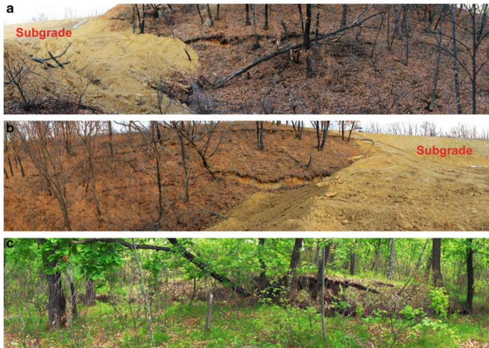
Fig. 8 Surface crack development at section A. (a) Crack in the south of the section A. (b) Crack in the north of the section A. (c) Landslide frontier at section A
