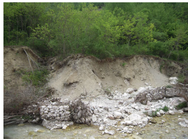
Fig. 3 Erosion of bank
