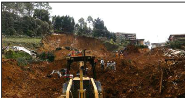
Fig. 3 Landslide at Alto Verde condominium
