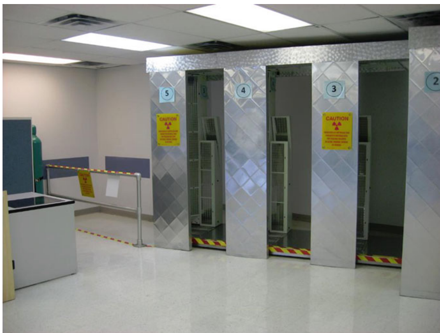
Fig. 6.15 Series of PCMs positioned at the primary RCA exit point. The RCA access control office is located immediately adjacent to the PCMs (Courtesy of Progress Energy Incorporated)
