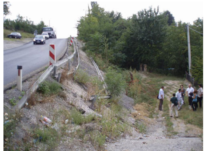
Fig. 5 Deformation on road M-19
