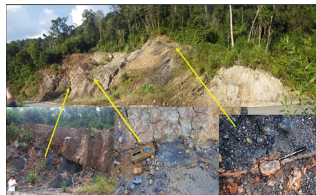
Fig. 10 Coal layer, landslide No. 21
