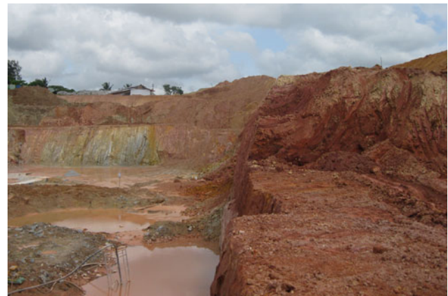
Fig. 2 Deep earth cutting sections in residual soils at Zone 2; Akuregoda, Colombo District
