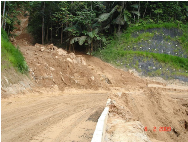
Fig. 8 The damage at FT 55 from Gap to Raub on 6 February 2009
