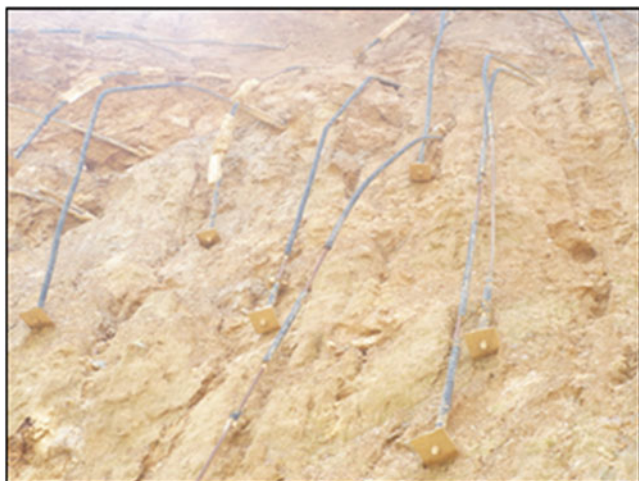
Fig. 3 Steel reinforcement hanging down from a failed soil nail system
