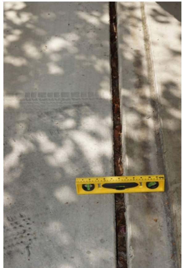
Fig. 7 Separation of garage slab from the driveway—identified during the field visit
