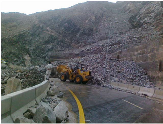
Fig. 3 One of the debris flows took place at the Al-Hada descent road
