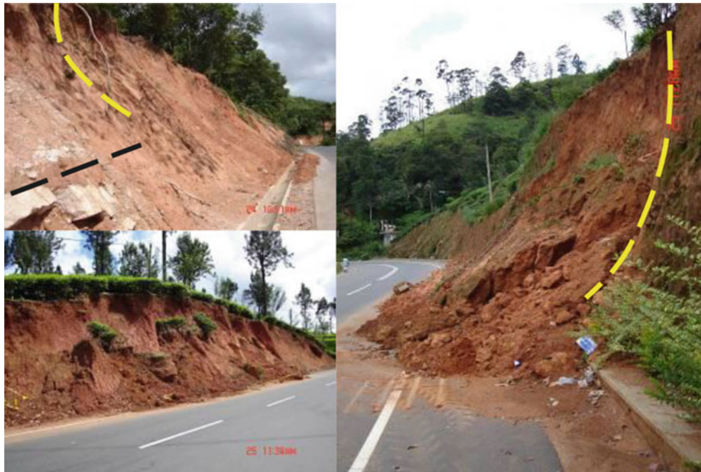
Fig. 8 Some typical examples of unsupported soil slump failures in residual soil exposed to surface saturation during rain
