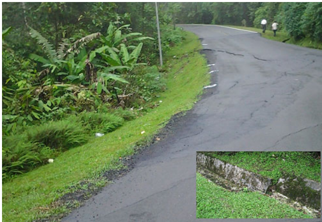
Fig. 8 Surface cracks (inset showing a displaced channel)
