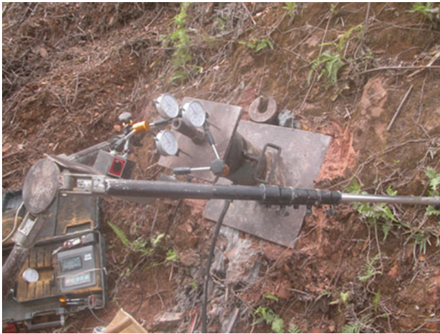
Fig. 9 Set up of in situ pullout test on hybrid V-armed flip anchor without grout at Dabong, Malaysia, 2012
