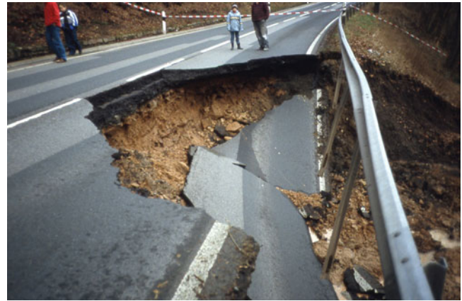
Fig. 3 Typical landslide damage to federal roads in the Lower Saxon Uplands (NW Germany) that caused repair costs of about $210,000 (in 2013 values) in the year 2003
