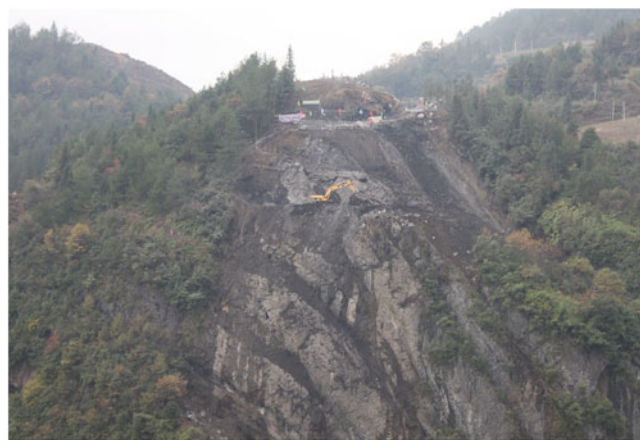
Fig. 2 Observed rock mass structures in the natural slope at the location of the No.5 arch abutment of Longqiao Bridge. Bedding planes show varying orientation. Natural slope height is 213 m
