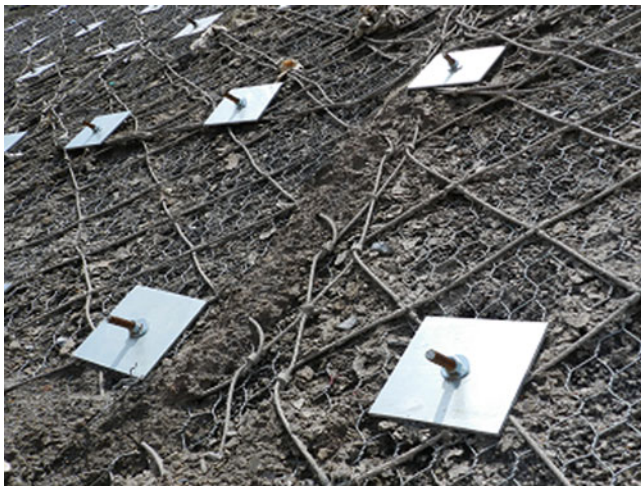
Fig. 6 Cable netting with erosion control synthetic mat tied down to the ground at the nail points
