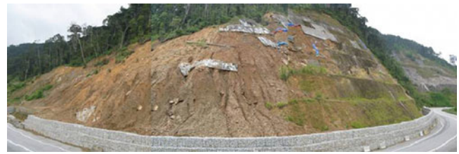
Fig. 1 Overview of slope at 46th km, Simpang Pulai—Kuala Berang Highway
