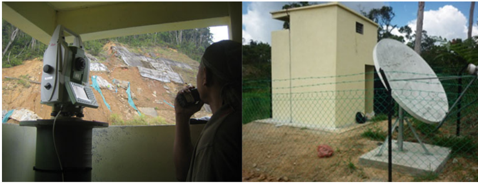
Fig. 3 Setup of robotic total station ( left ), and antenna for satellite communications ( right )
