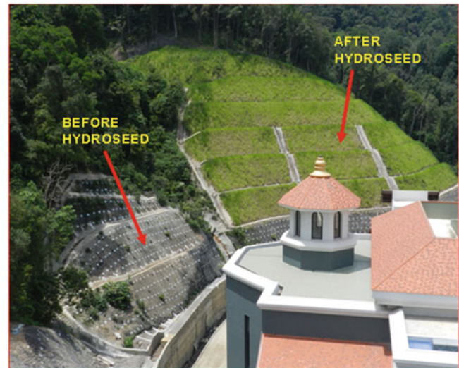
Fig. 7 Application of cable netting and erosion control synthetic mat before and after hydroseeding
