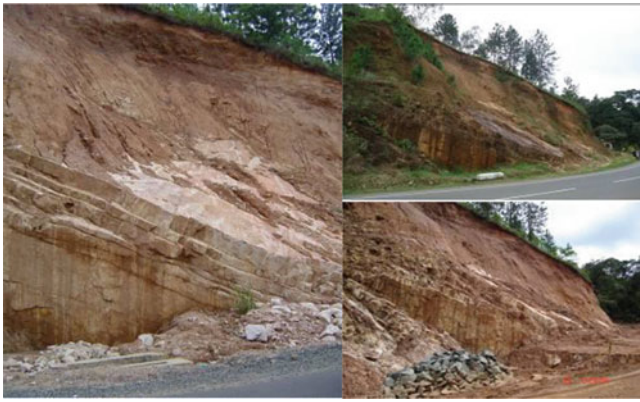
Fig. 14 Geologically unstable rock-soil slope condition
