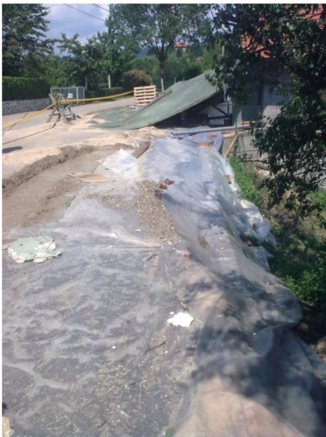
Fig. 1 Picture of the terrain slope with part of the damaged road
