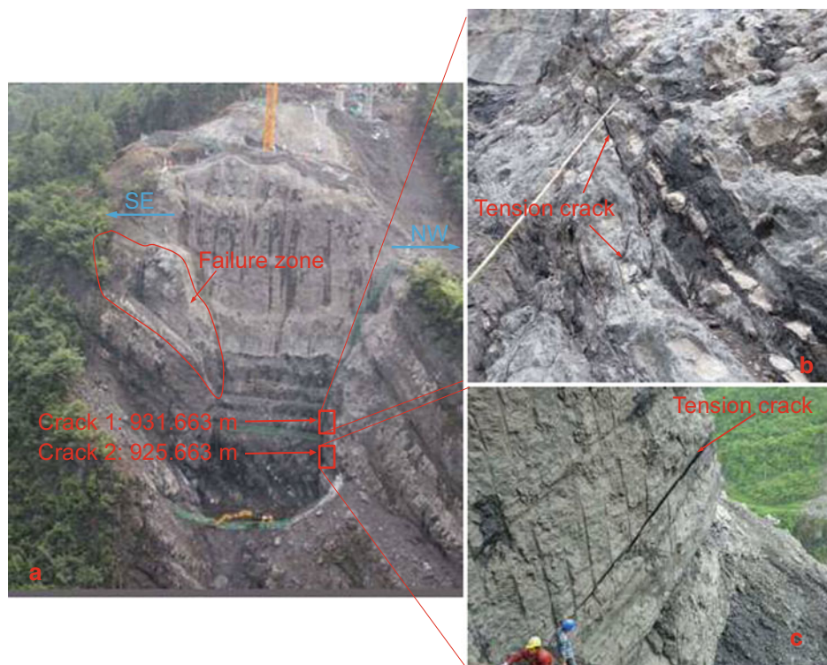
Fig. 8 Rock slope deformation and failure due to excavation of the No.5 arch abutment foundation pit. (a) The SE slope slid along bedding planes and the NW slope showed minor flexural toppling on bedding when the excavation had reached elevations of 943 m and 919.663 m, respectively. Tension cracks 1 and 2 opened along bedding planes at
