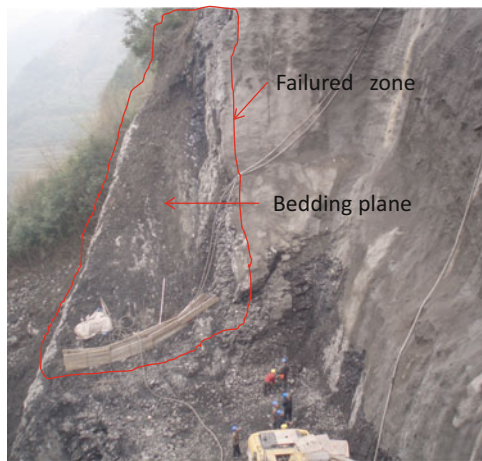
Fig. 7 Sliding failure of the SE slope occurred along a bedding plane when the arch abutment foundation pit had been excavated to an elevation level of 943 m.
