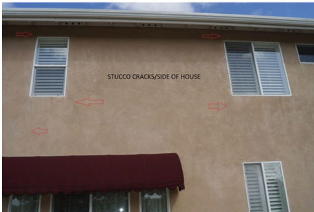
Fig. 4 Cracks on the stucco of the building
