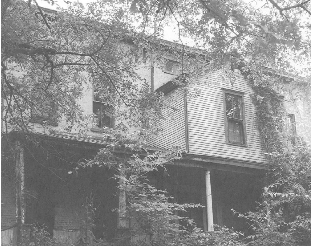
FIG. 4— Historic buildings on overgrown sites will deteriorate rapidly as moisture penetrates through damaged exteriors. In this view, vines have attached themselves to the house, keeping moisture in contact with deteriorating surfaces; gutters have been pulled off the porch; missing downspouts have caused mortar to erode; and broken glass allows driving rain to penetrate the interior. Photo: NPS files.
