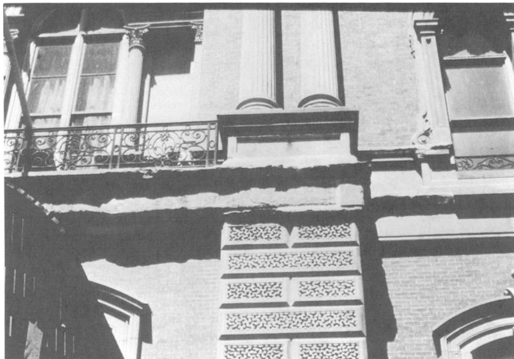
FIG. 11—Some repair treatments will result in damage more serious than the original deterioration. Synthetic patching compounds were used to repair deteriorated sandstone, only to fail within a few seasons. Moisture trapped behind the synthetic waterproof patches deteriorated sound stone and the patches failed. Deteriorated features should be replaced with the original materials to the extent possible. If substitute materials are used, they should work within the expansion, contraction, and permeability properties of the original materials. Photo: NPS files.
