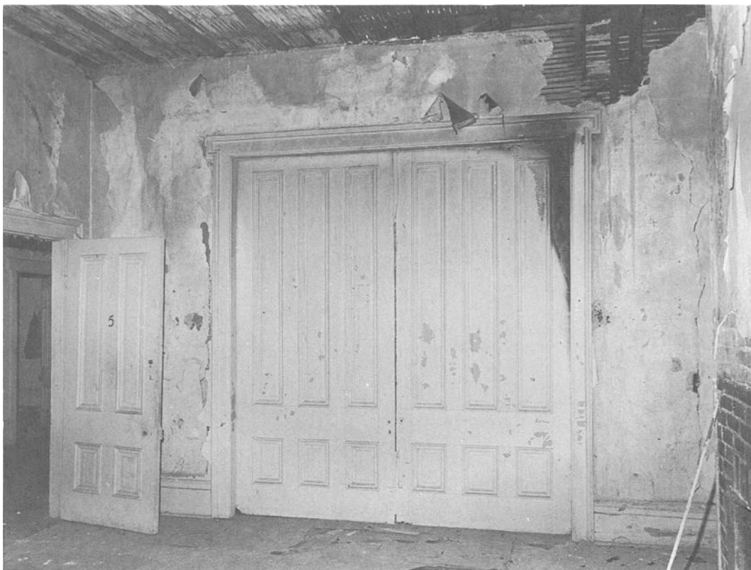
FIG. 17—The damage to this historic plaster was in part the result of moisture used to put out a serious fire. Once plaster interiors are saturated with water, they must be slowly and thoroughly dried out before effective repairs can be made. For plastered walls, this drying out process may take several months and the movement of air may be more beneficial than the use of heat. Rapid drying with heat often causes wooden elements to crack on the surface, still leaving moisture in the walls behind. Once dried, these lath walls will take fresh plaster, and they should not be covered with modern drywall. Photo: NPS Files.
