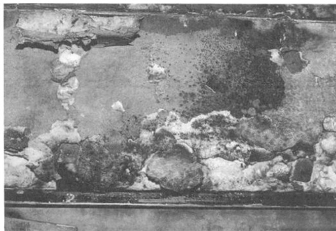
FIG. 3— Cladosporium and other fungi contaminating sound lining in an air handling system.
