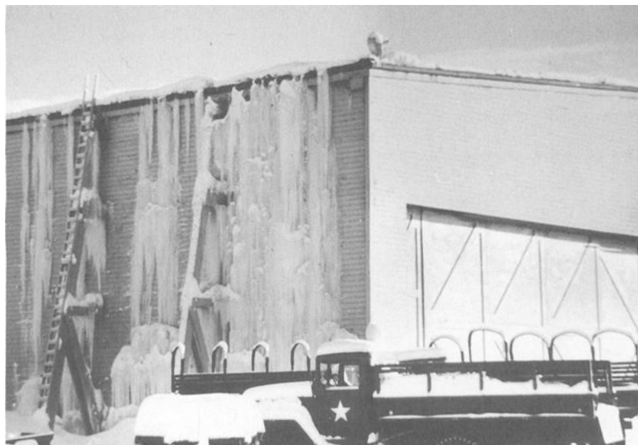
FIG. 28—Icings can form on walls if the eaves do not overhang far enough.
