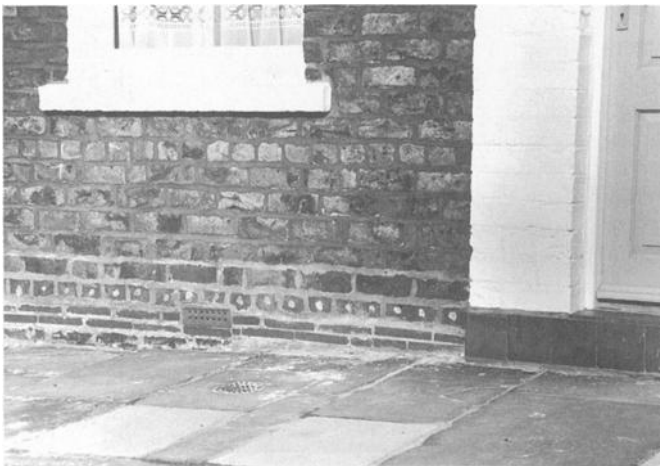
FIG. 7—Not all methods of dealing with rising damp are successful. Chemicals injected through the exterior walls to create a waterproof barrier can be visually disfiguring and often are not effective in curing rising damp. These treatments should be considered only as a last resort and injection should be from the interior to avoid disfiguring the building exterior. Photo: NPS Files.
