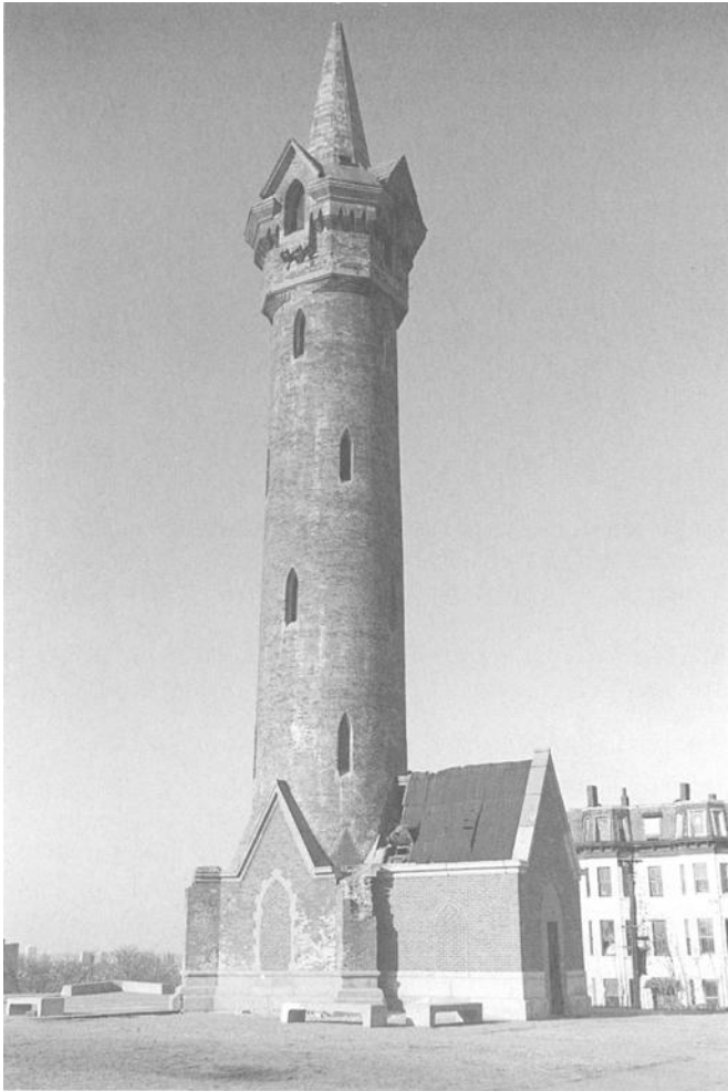
FIG. 13—Rapid deterioration of a historic building occurs when the roof is not maintained. In this unoccupied observatory tower, the temporary roof over the entrance has failed, allowing moisture free access to the interior. Note the efflorescence caused by this moisture and the loss of masonry at the side buttress. Photo: courtesy SPNEA, NPS files.
