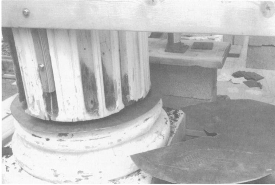
FIG. 6—Moisture rising through foundations is often difficult to treat. In some cases the insertion of a physical barrier may help stop capillary action. This wooden replacement column, only 15 years old, was showing rapid decay (dark stains) as a result of moisture at the stone base. To arrest further deterioration, lead sheets were inserted to prevent rising damp. Photo: Bryan Blundell.
