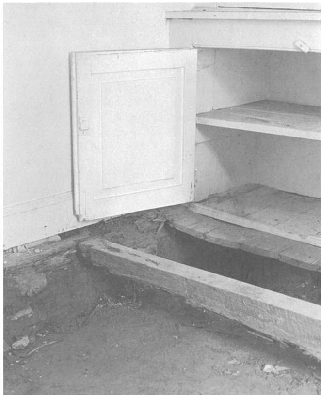
FIG. 14— Moisture can cause dry rot, a type of fungus, to structurally weaken framing members. These floor joists have been in contact with wet foundations just above a damp crawl space. The new replacement joist should be isolated from these moist conditions, perhaps by excavating the crawl space to a deeper depth, by adding a vapor barrier over the dirt layer, and by increasing the natural ventilation in the crawl space. Photo: NPS files.
