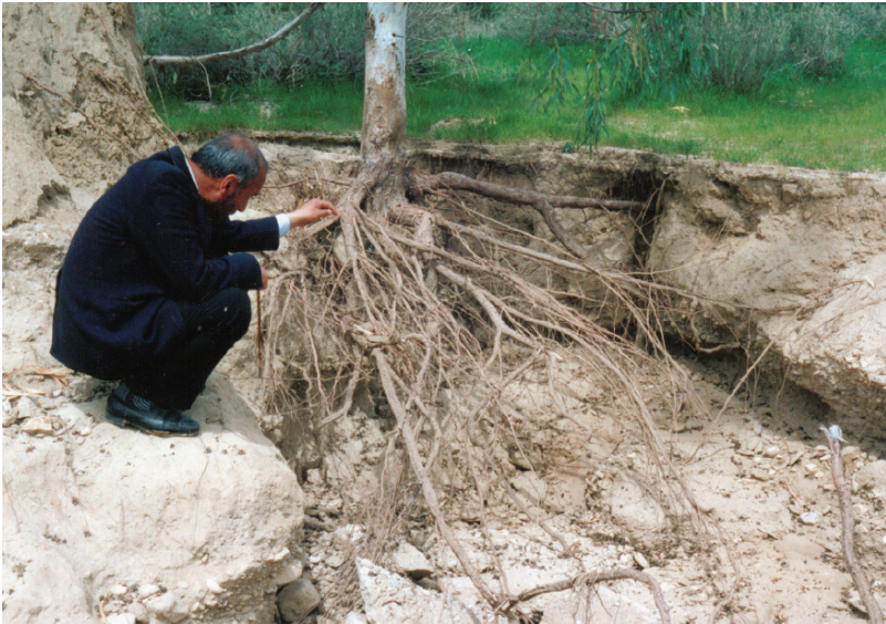
Fig. 2 Copious growth of eucalyptus roots has undermined a masonry chute. The minimum distance between a Eucalyptus camaldulensis Dehnh. tree and a solid chute should be 10m.
