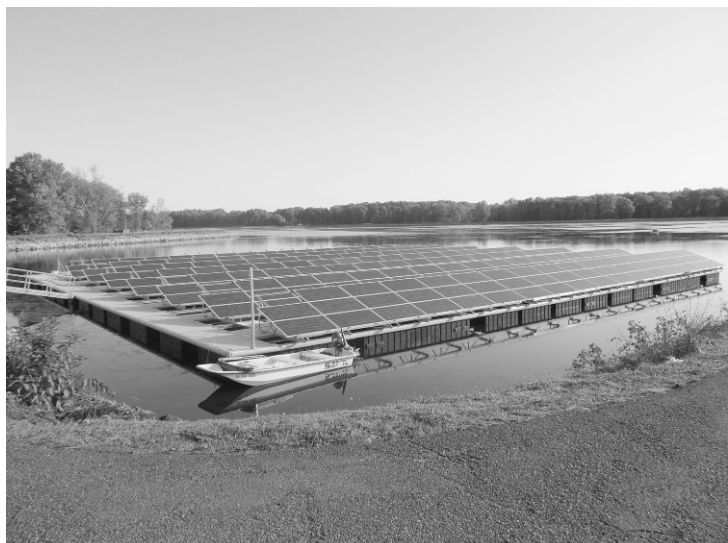
Figure 3-2. Floating photovoltaic arrays, Canoe Brook Water Treatment Plant, Millburn, New Jersey. (Courtesy of American Water.)
