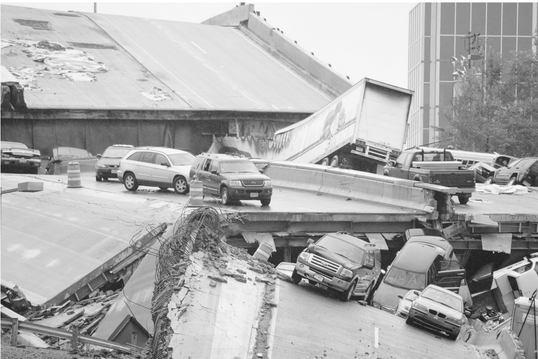
Figure 1-1. Cars remain on the collapsed portion of I-35W Mississippi River Bridge, in Minneapolis, Minnesota, four days after the August 2007 collapse. (Courtesy of Kevin Rofidal, US Coast Guard.)
