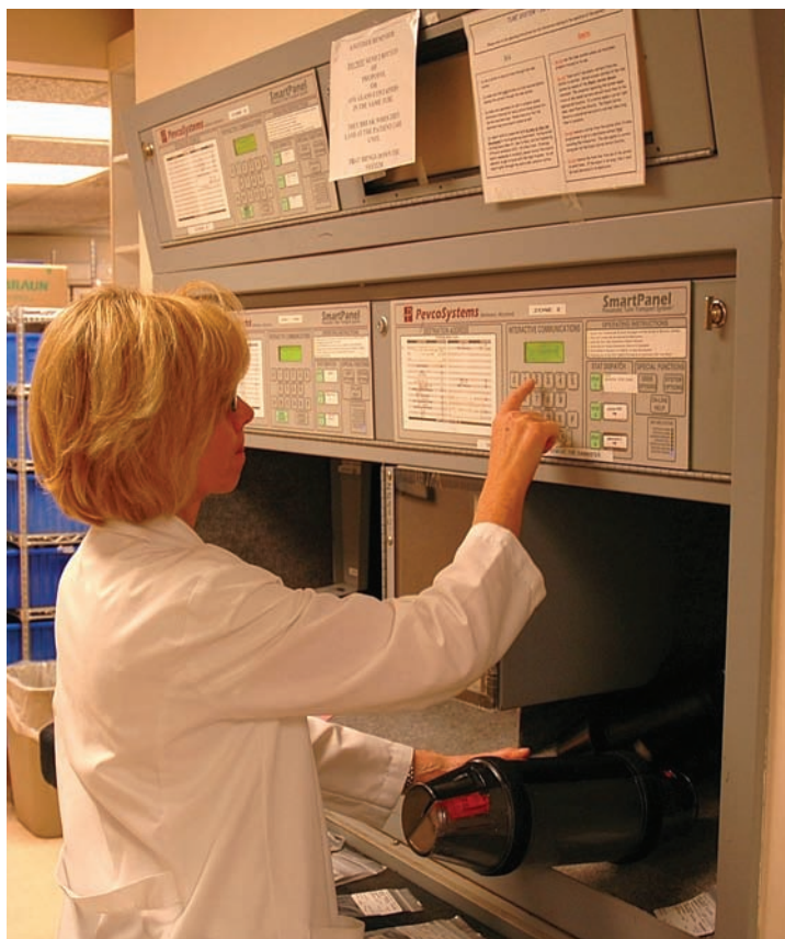
FIGURE 18-4 Pneumatic tube system.
