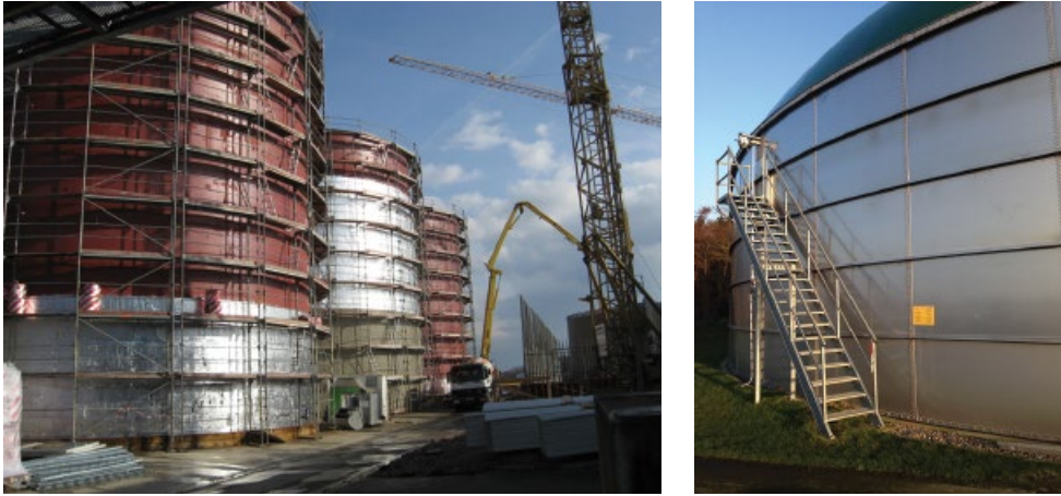
Figure 6.62 Biogas digesters of welded and coated carbon steel (left photo: © Schachtbau Nordhausen GmbH) and bolted, stainless steel.
