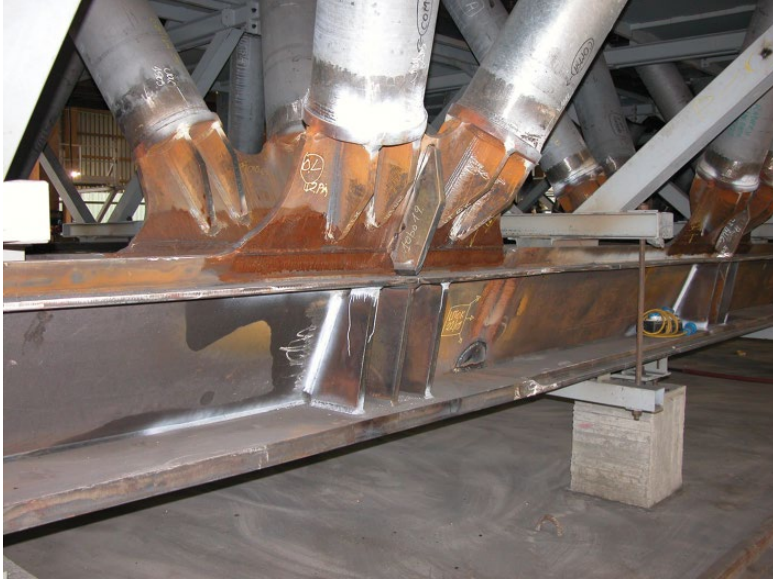
Figure 2 To maximise the simplicity and easiness of fabrication of the inferior nodes, nine alternatives were compared. © MCA Engineering.
