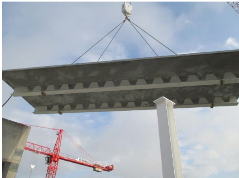
Figure 4.19 Spanning a building without columns using a TOPfloor INTEGRAL composite deck – view of underside of deck and installation of element. © H. Wetter AG, CH-Stetten.
