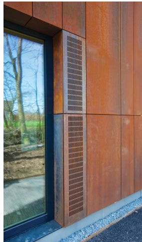
Figure 2 Detail of the ventilation system next to the window. © Gilles Martin.
