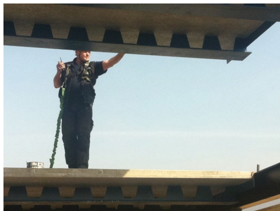
Figure 4 Construction phase – rapid construction with prefabricated TOPfloor INTEGRAL elements. © H. Wetter AG.
