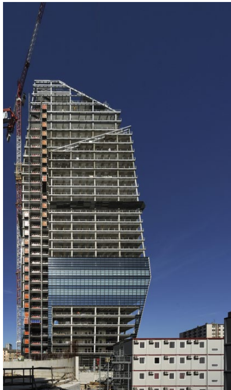
Figure 3 Construction phase – the steel structure is already finished. © Oskar Da Riz / Stahlbau Pichler.
