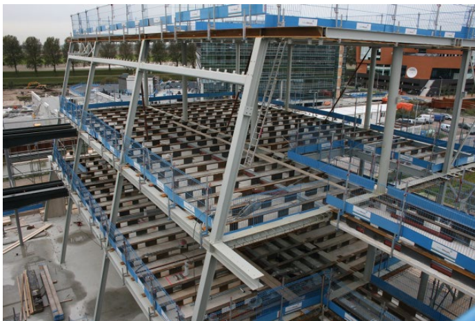
Figure 2 During the construction phase – the hole pattern in the steel beams of the Slimline floor system for accommodation of all common building installations is still visible. © Slimline Buildings.
