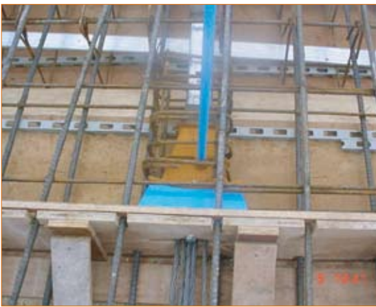
Figure 7.38 Bursting reinforcement for a typical live end in a post-tensioned slab (courtesy of Sir Robert McAlpine Ltd)
