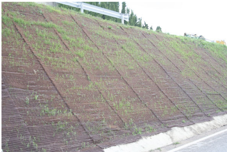
Fig. 5.10 View of the use of seeds to control soil losses on road embankments (Photo: A Cerdà)
