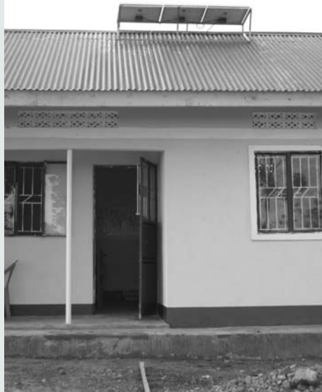
Figure SH8.1 Appropriate Technology: Photovoltaic panels that were sourced locally and installed using local labor in a rural Ugandan village.
