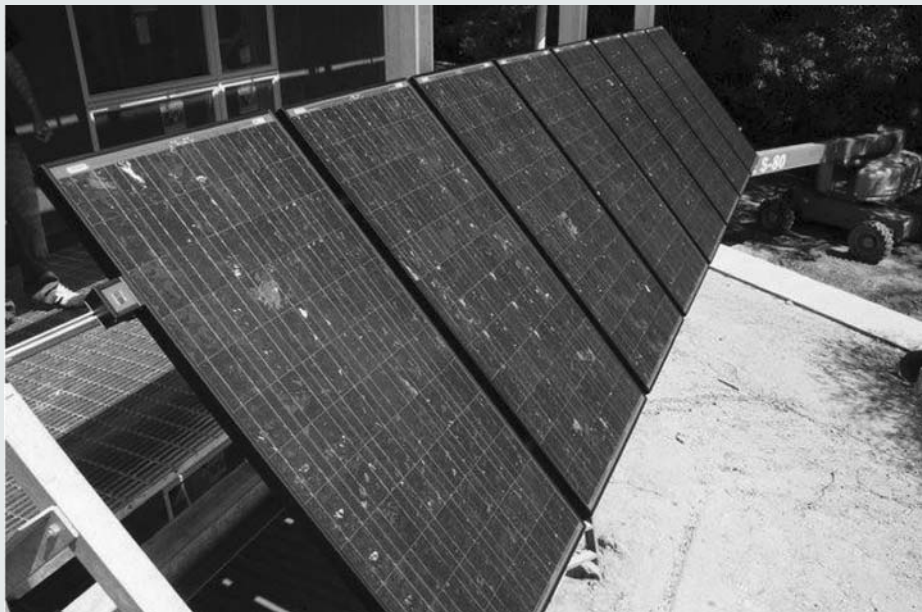
Figure S.1.3 Photovoltaic panels at the Home Depot Smart Home at Duke University.
