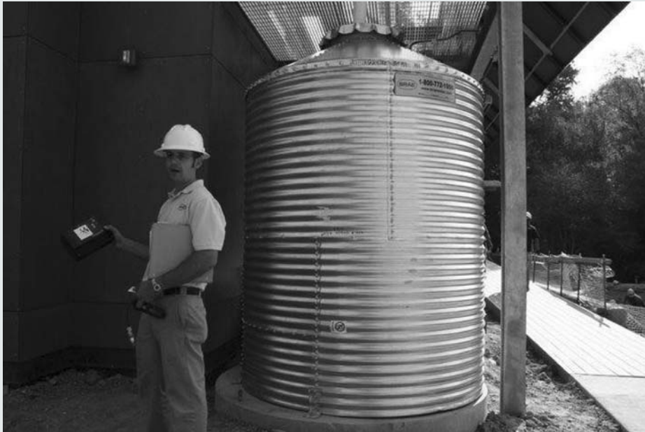
Figure S.1.2 A 1000-gallon rainwater cistern at the Home Depot Smart Home at Duke University.
