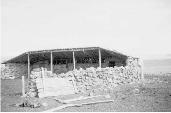
Figure 5.2 A herder does summer repair work on a winter livestock shelter, South Gobi Aimag, 2006.
