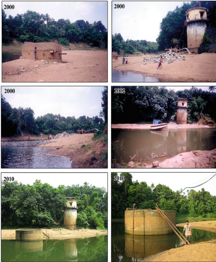
Plate 4.8 Impact of sand mining on rural water supply schemes: a A water intake structure is exposed due to river bed lowering; b Direct pumping of water into the newly constructed intake pit; c A check dam constructed for raising water level in the river reach; d Tilting of the water intake due to uncontrolled sand mining; e and f The lowered river channel and the newly constructed water intake structure for the rural water supply scheme
