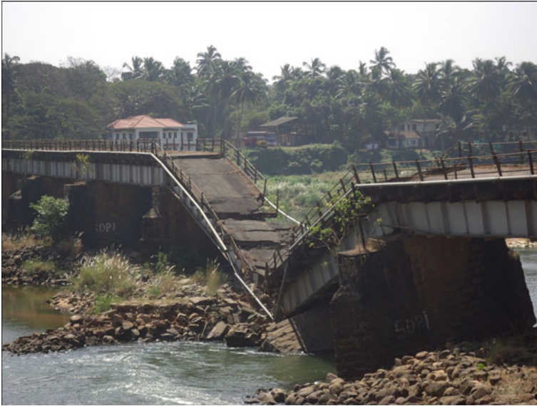
Plate 4.2 Collapse of bridge in Bharathapuzha river (SW India) near Shornur due to channel incision
