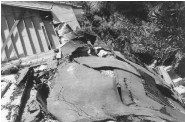
FIGURE 10.32 Laguna Niguel landslide: another view of the toe of the landslide where the road has been uplifted 20 ft.
