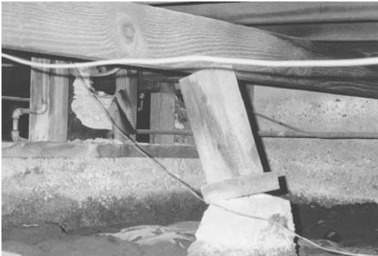
FIGURE 9.23 Expansive soil damage of a raised wood floor foundation. Note the wet condition of the soil in the crawl space.
