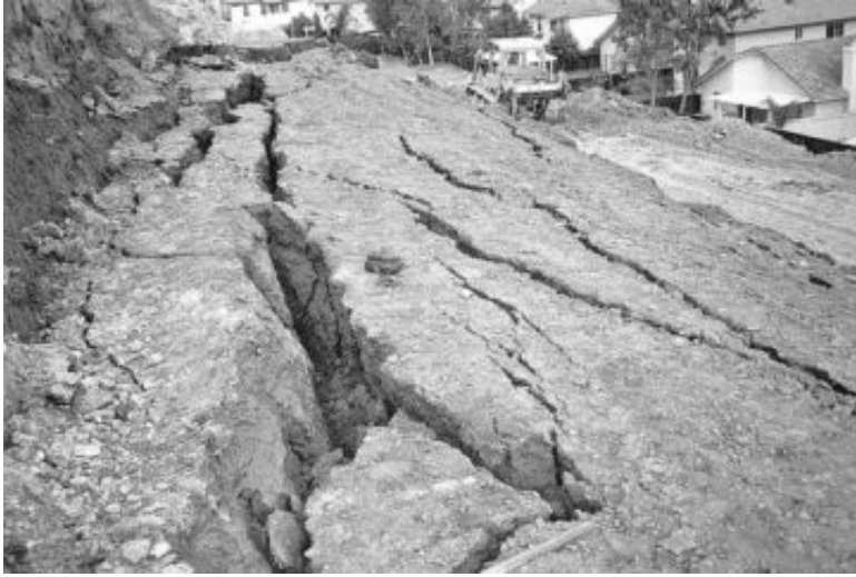
FIGURE 16.1 Slope failure during the grading of a site. The backpack located in the middle of the photograph provides a scale for the size of the ground cracks.
