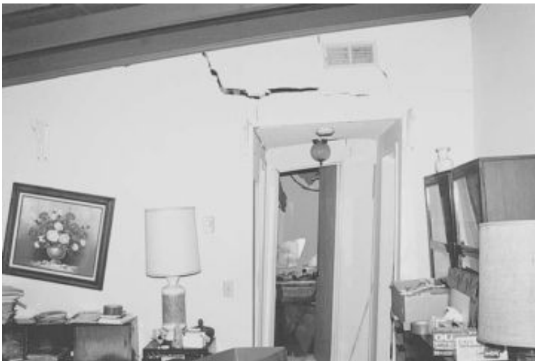
FIGURE 10.8 Damage to interior wallboard and distortion of door frames.
