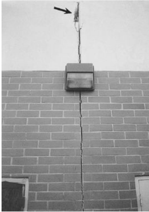
FIGURE 10.3 Joint separation between wall panels.
