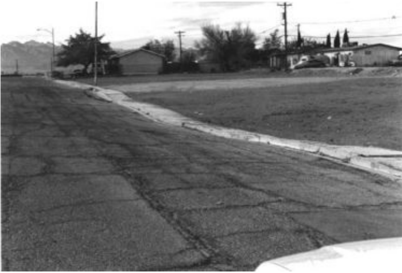
FIGURE 7.20 Settlement of the street and sidewalk due to ground fissures, Las Vegas, Nevada.
