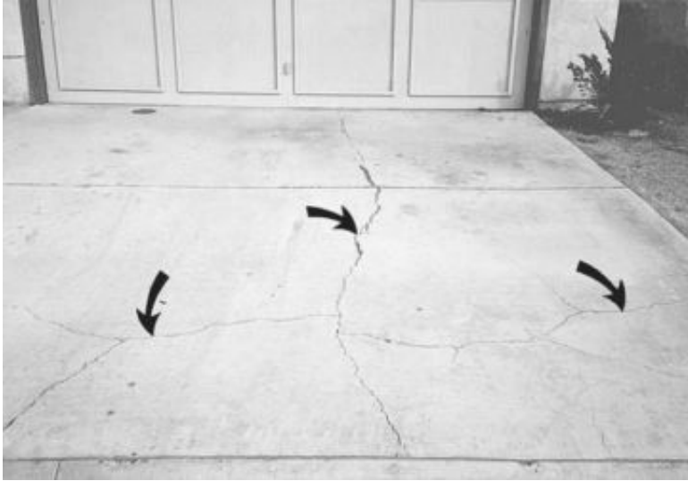
FIGURE 9.31 Driveway cracking due to expansive soil.
