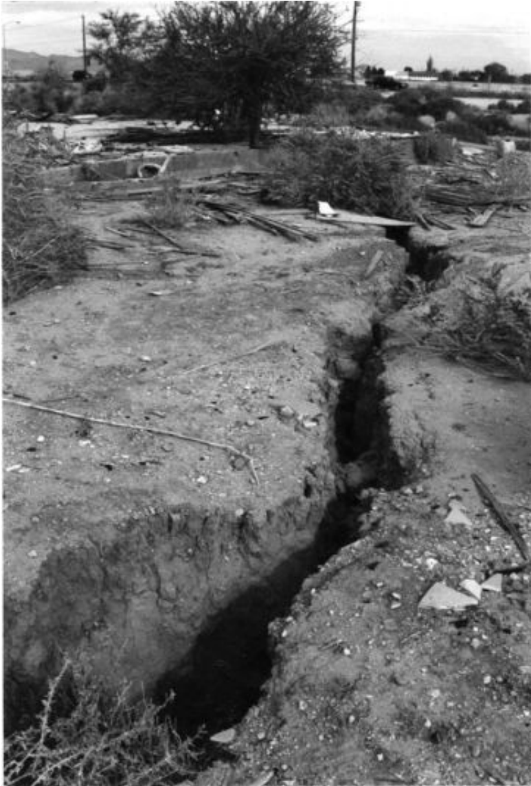
FIGURE 7.17 Ground fissure in Las Vegas, Nevada.
