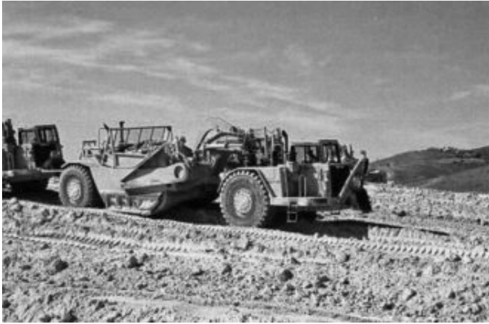
FIGURE 15.10 The scraper is used to excavate material from the borrow area, transport it to the site, dump it at the site, and then compact the soil.
