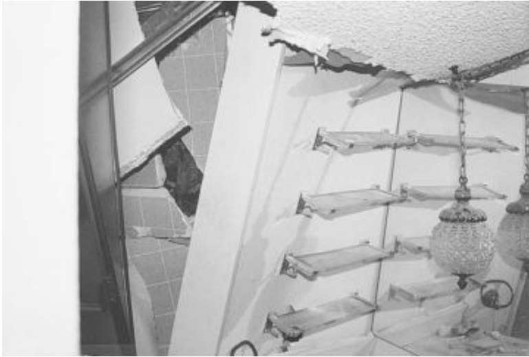
FIGURE 10.7 Damage to bathroom.
