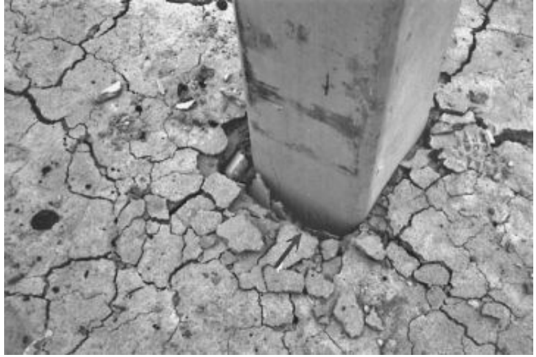
FIGURE 16.25 This prestressed concrete pile struck an underground obstruction, displaced laterally, and broke near ground surface. The arrow points to the location of the breakage.
