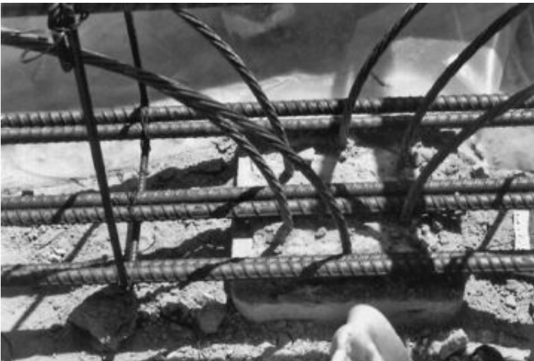
FIGURE 16.30 Close-up view of the top of a prestressed pile with the steel reinforcement from the grade beam positioned on top of the pile. The strands from the pile are attached to the steel reinforcement in the grade beam.
