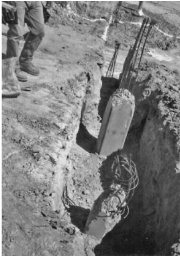
FIGURE 16.27 The prestressed concrete pile at the bottom of the picture is the same pile shown in Fig. 16.25. The pile near the center of the photograph is the replacement pile. The broken pile and the replacement pile will be attached to the grade beam.
