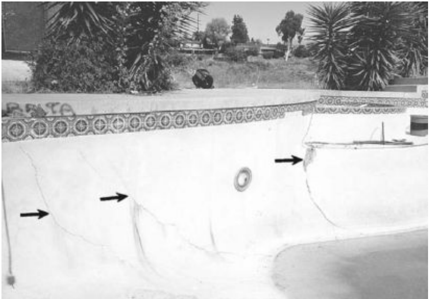
FIGURE 7.5 Damage to a pool shell due to collapse of underlying uncompacted fill (arrows point to cracks in the pool shell).
