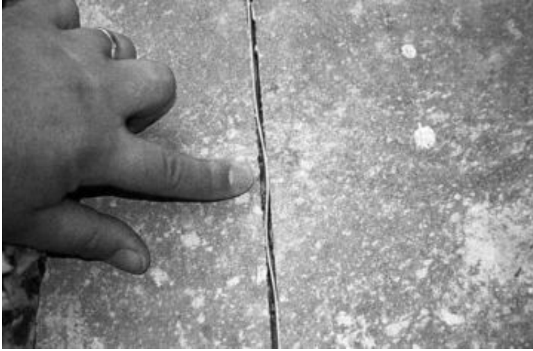
FIGURE 12.14 View of a plastic strip that was used to form a contraction joint. The plastic strip is sometimes referred to as a zip-strip . The gaps that have opened-up on both sides of the plastic strip were caused by drying shrinkage.
