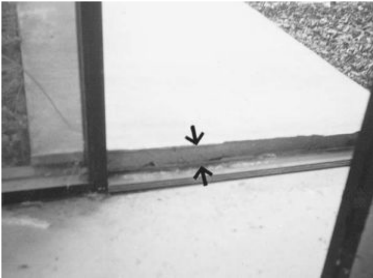
FIGURE 9.30 Sidewalk uplift due to expansive soil.
