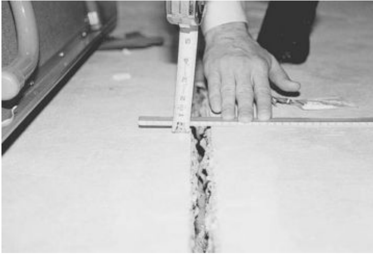
FIGURE 10.2 Damage due to lateral movement.
