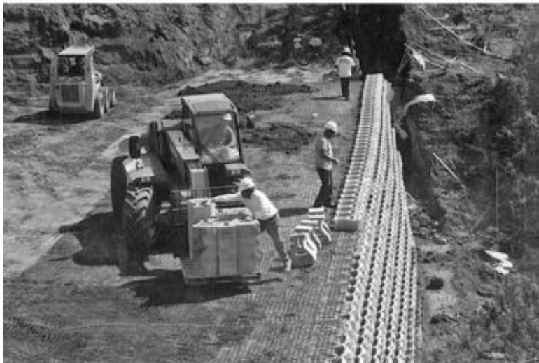
FIGURE 11.10 Two views of the installation of the geogrid for a mechanically stabilized earth retaining wall. The large arrows indicate the width of the mechanically stabilized zone and the small arrow points to a geogrid splice.
