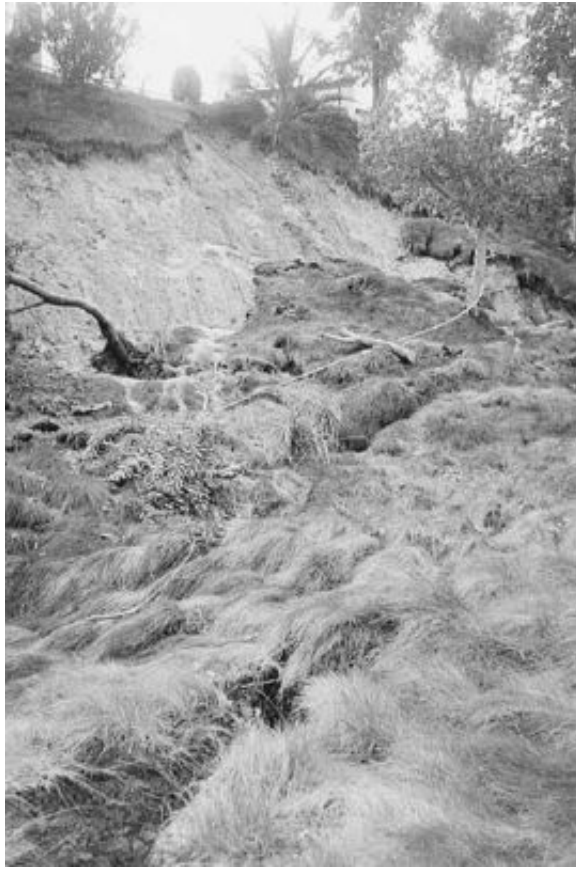
FIGURE 10.13 Surficial slope failure in a fill slope.
