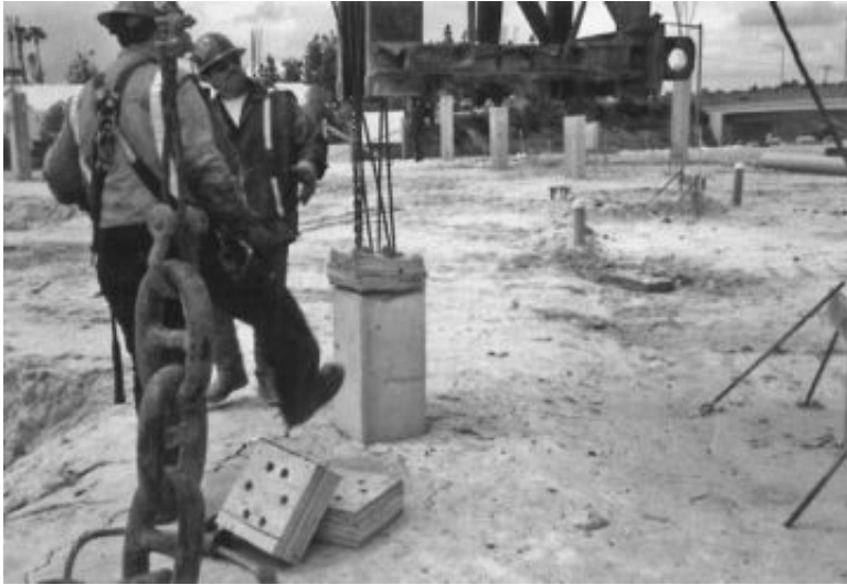
FIGURE 16.23 A prestressed concrete pile has been successfully driven to the bearing strata. The wood block shown on the top of the concrete pile was used as a cushion in order to protect the pile top from being crushed during the driving operation.
