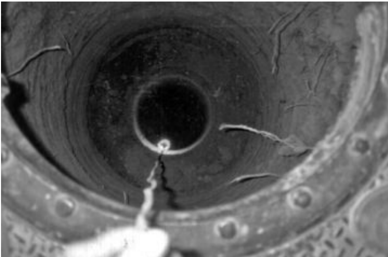
FIGURE 16.12 A light has been lowered to the bottom of the pier in order to observe embedment conditions.
