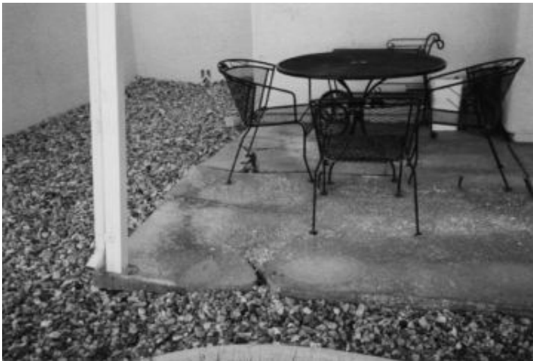
FIGURE 12.1 Sulfate attack of a concrete patio.
