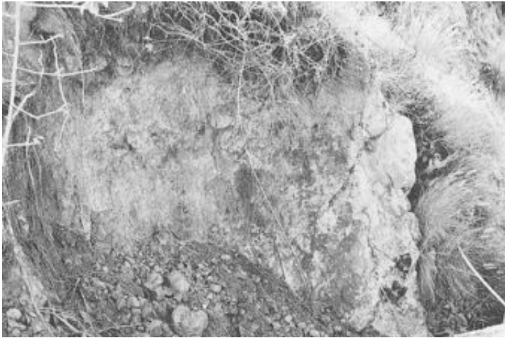
FIGURE 10.5 Location of rockfall.
