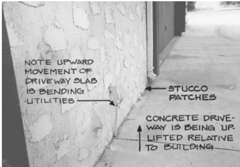
FIGURE 9.32 Concrete flatwork uplifted by expansive soil.
