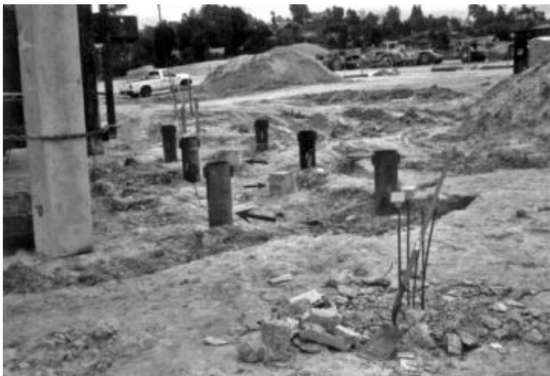
FIGURE 16.32 Pile load test. The small arrows point to the prestressed concrete piles that will be subjected to a load test. The large arrow points to one of the six anchor piles.
