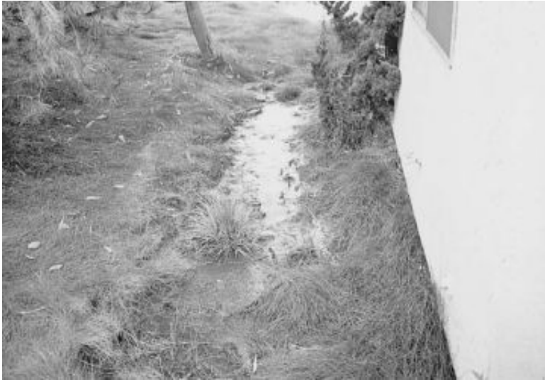
FIGURE 12.21 Poor surface drainage at a condominium complex.
