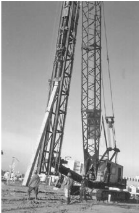
FIGURE 16.22 Pile driving equipment. A prestressed concrete pile is in the process of being hoisted into position.
