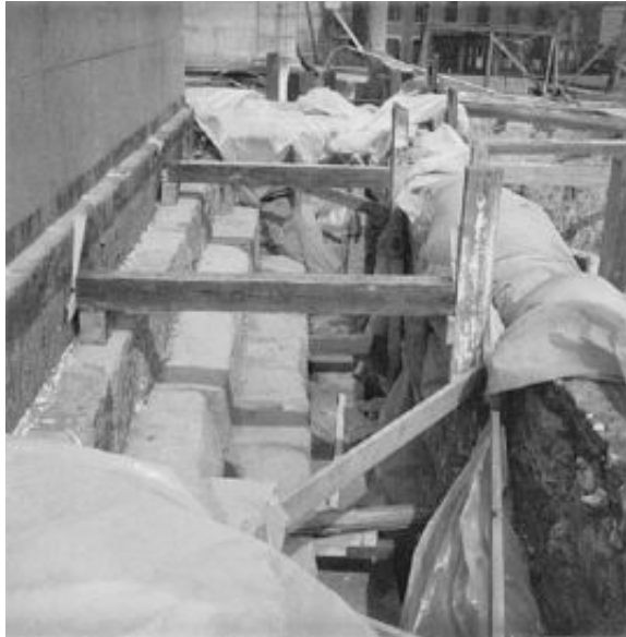
FIGURE 12.5 Exposed foundation of the Bunker Hill Monument.
