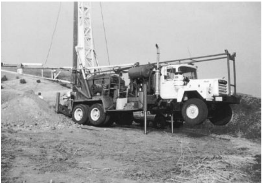
FIGURE 2.4 A flight auger drill rig (top) and a bucket auger drill rig (bottom).
