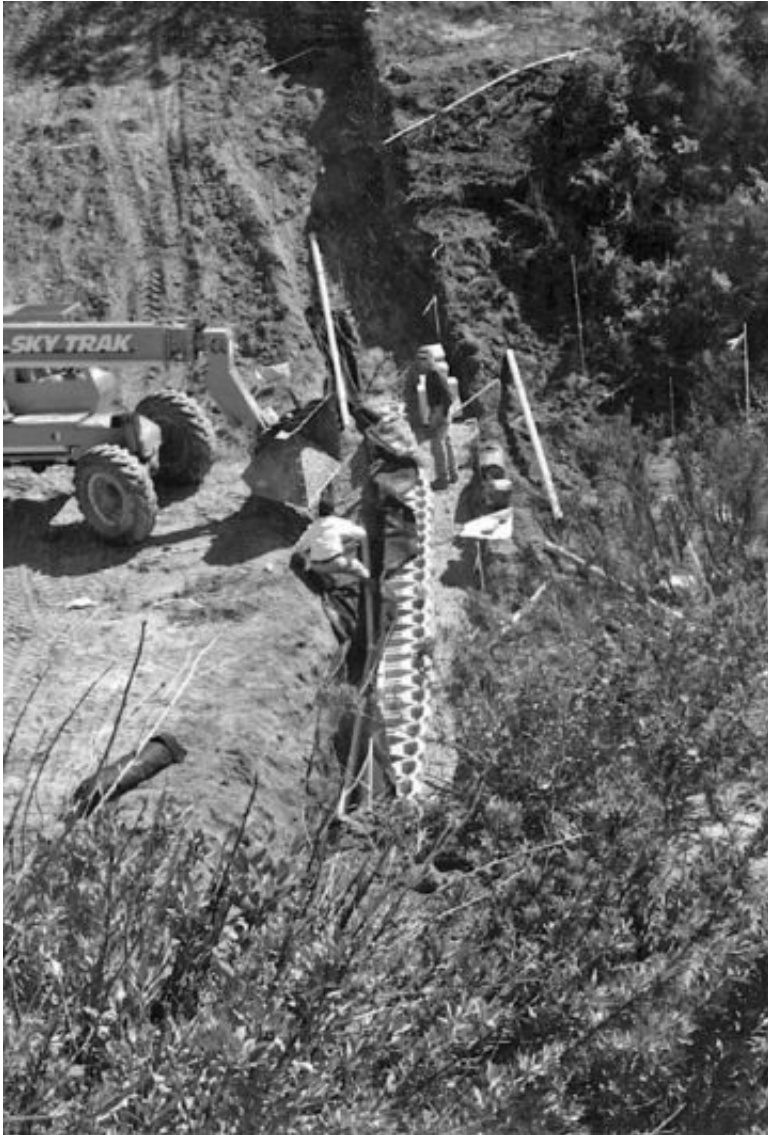
FIGURE 11.9 Excavation of key and installation of drainage system for a mechanically stabilized earth retaining wall.
