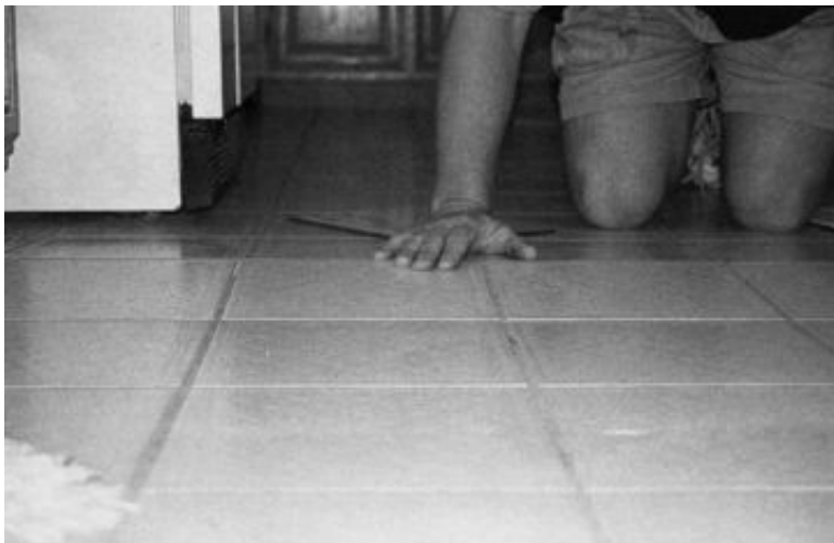
FIGURE 12.18 Uplift of floor tile due to moisture migration through a crack in the slab-on-grade foundation. The floor tile absorbed moisture and expanded, resulting in the uplift shown in the photograph.
