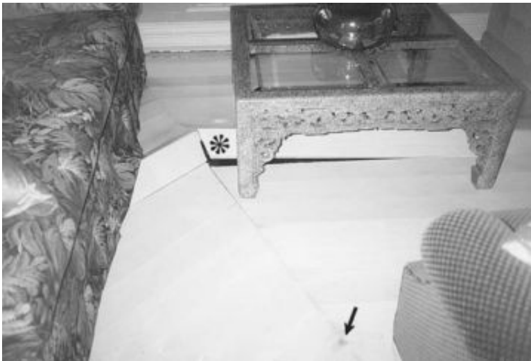
FIGURE 12.17 Damage to wood flooring. The arrow points to a moisture stain and the asterisk indicates upward warping of the wood floor.
