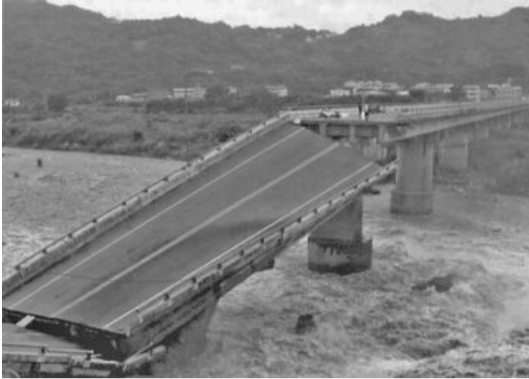
FIGURE 13.5 Collapsed bridge north of Fengyuen caused by surface fault rupture associated with the Chi-chi (Taiwan) earthquake on September 21, 1999. (Photograph from the USGS Earthquake Hazards Program, NEIC, Denver.)
