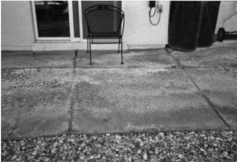
FIGURE 12.2 Another example of sulfate attack of a concrete patio.
