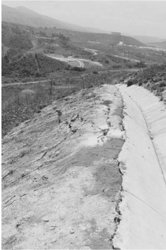
FIGURE 10.15 Ground cracks associated with incipient surficial instability.
