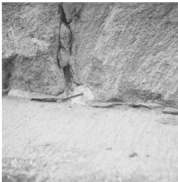
FIGURE 12.6 Deteriorated mortar between the granite blocks of the Bunker Hill Monument foundation.
