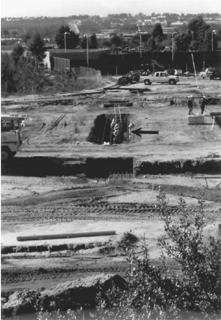
FIGURE 16.3 Installation of steel reinforcement in footings. The arrow points to the workers in the footing excavation in the process of installing the steel reinforcement.
