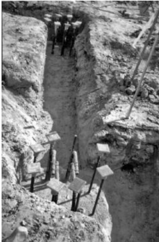
FIGURE 16.14 Excavation for the grade beam that will span between the two piers.
