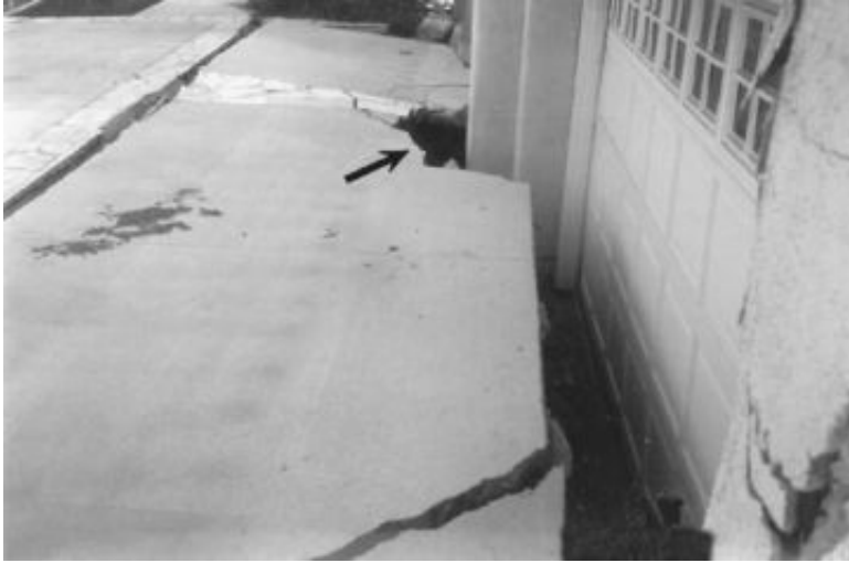
FIGURE 10.37 Laguna Niguel landslide: head of the landslide where a house has dropped downward. (Note: The arrow points to the area where the house foundation has punched through the driveway on its way down.)
