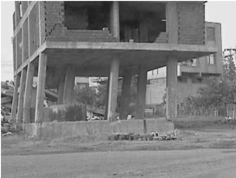
FIGURE 14.4 Damage caused by a soft story at the first-floor level. The damage occurred during the Kocaeli earthquake in Turkey on August 17, 1999. (Photograph by Mehmet Celebi, USGS.)
