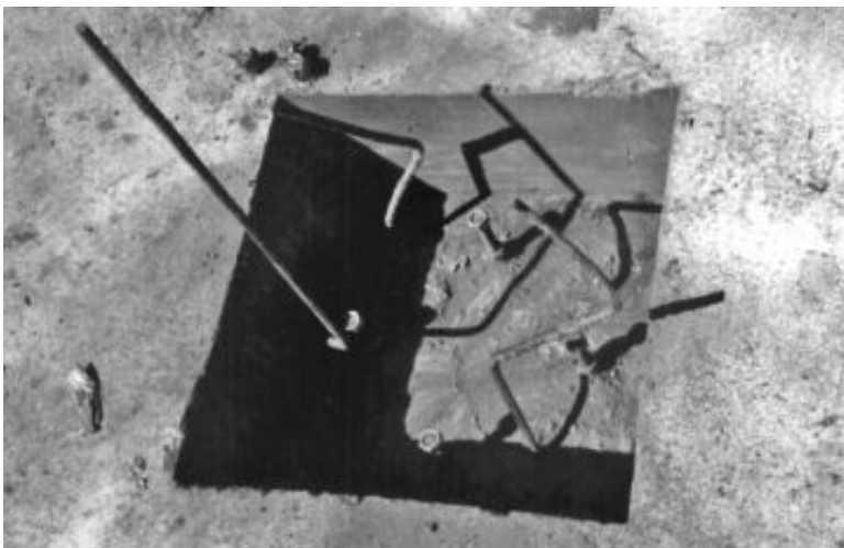
FIGURE 16.20 Location where a steel column will be attached to the top of a pier.
