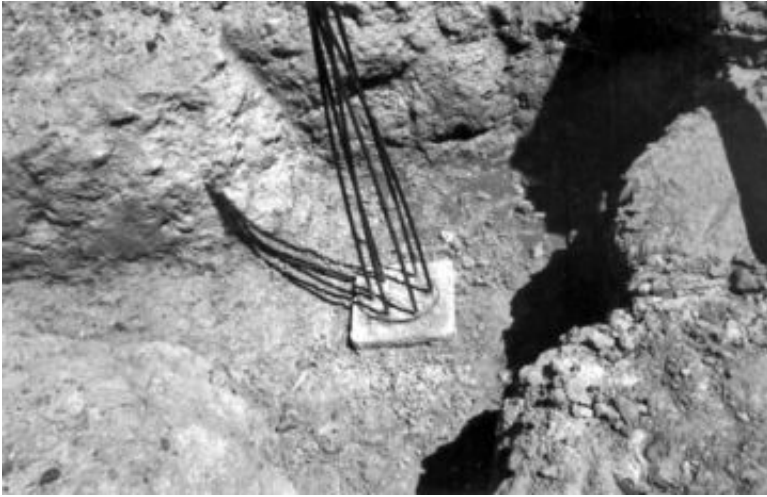
FIGURE 16.29 Close-up view of one of the prestressed piles showing a trimmed top surface with the strands extending out of the top of the pile.
