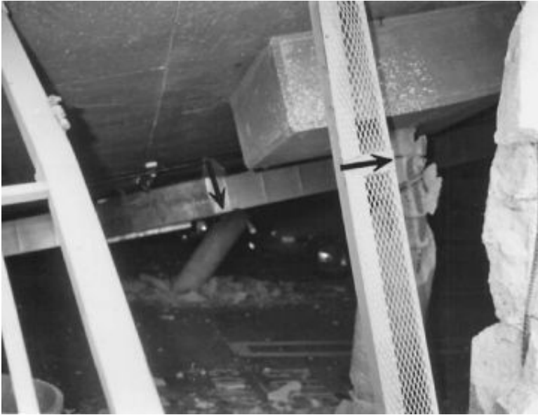
FIGURE 14.3 View inside the collapsed first floor parking garage (the arrows point to the columns). The building collapse occurred during the Northridge earthquake in California on January 17, 1994.
