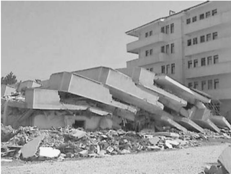
FIGURE 14.6 Pancaking of a building during the Kocaeli earthquake in Turkey on August 17, 1999. (Photograph by Mehmet Celebi, USGS.)
