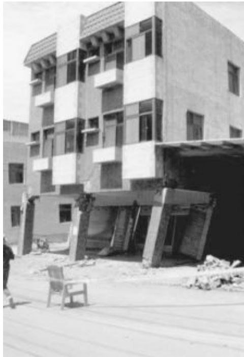
FIGURE 14.1 Damage due to a soft story at the ground floor. The damage occurred during the Chi-chi earthquake in Taiwan on September 21, 1999. (Photograph from the USGS Earthquake Hazards Program, NEIC, Denver.)
