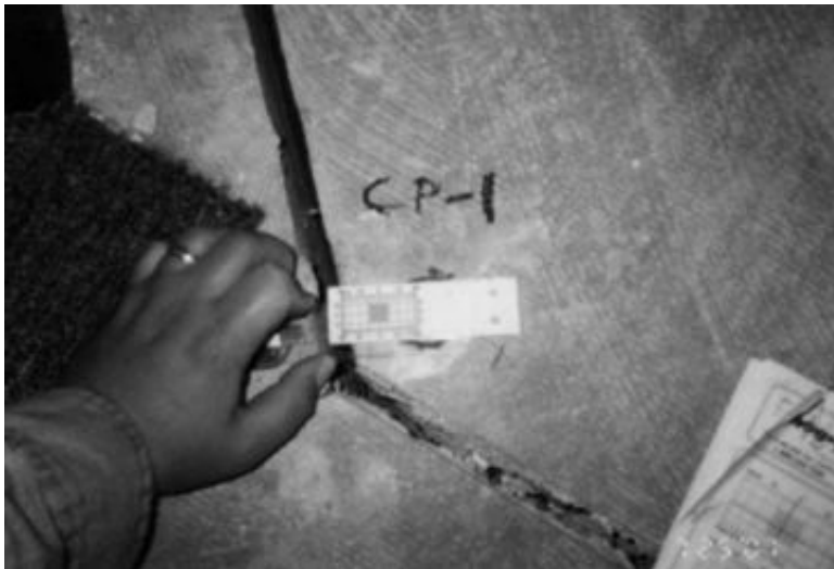
FIGURE 12.15 About 1 in. (25 mm) opening of a contraction joint due to slope movement that pulled apart the foundation at the contraction joints. A crack monitoring device has been placed across the contraction joint.
