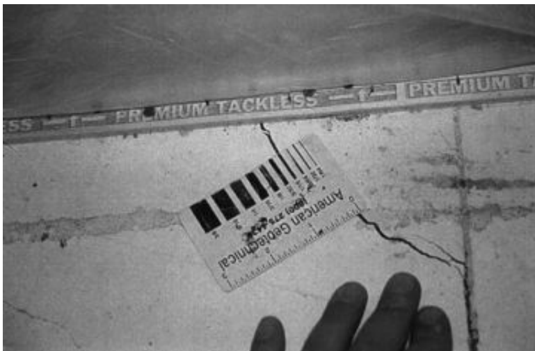
FIGURE 12.13 Concrete slab-on-grade having a contraction joint that was not saw-cut deep enough. Note how the slab crack deviates from the shallow saw-cut joint.
