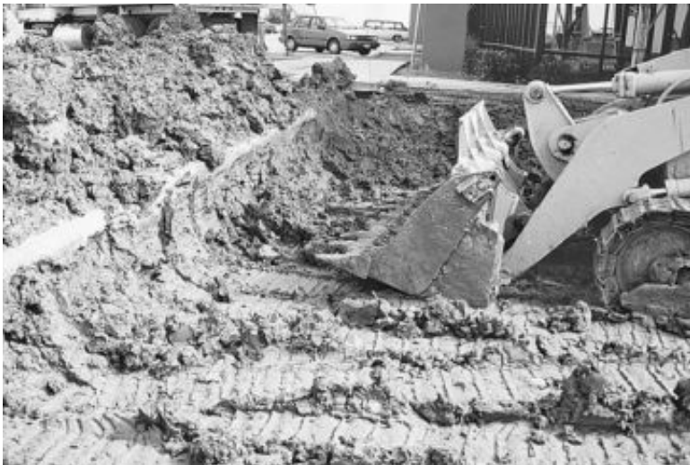
FIGURE 15.16 Pumping of clay subgrade during construction.
