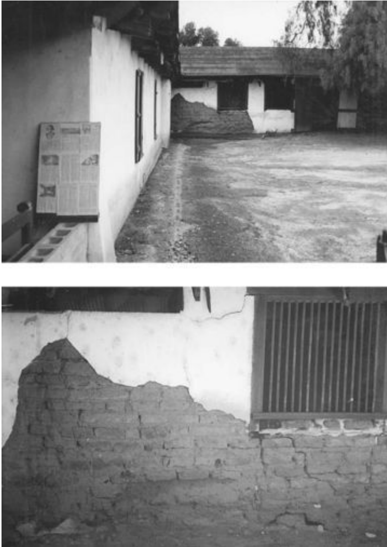
FIGURE 12.8 Deterioration of adobe. The lower photograph is a close-up view of the upper photograph. Note that the individual adobe blocks are visible in the lower photograph.
