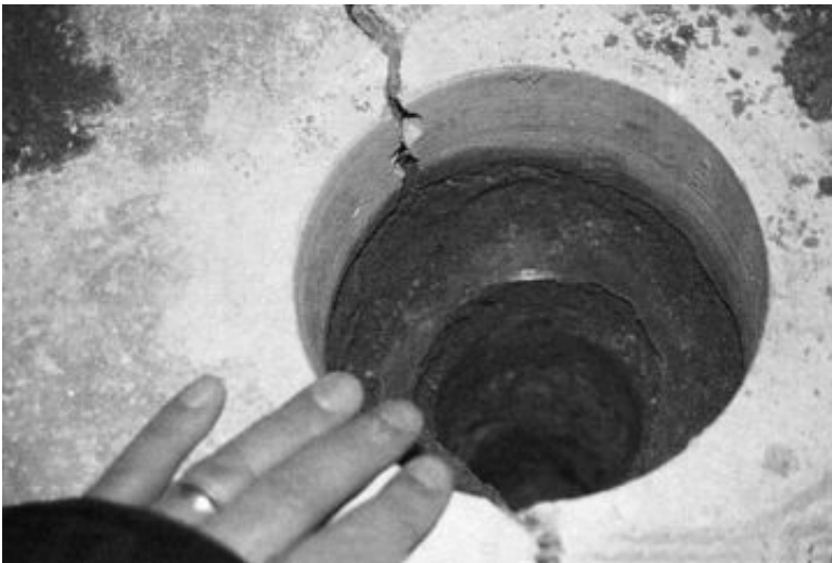
FIGURE 12.12 Excessive shrinkage crack in a concrete slab-on-grade foundation. The concrete has been cored and the crack is observed to penetrate the entire thickness of the concrete. Note that a visqueen moisture barrier is visible at the location of the core.
