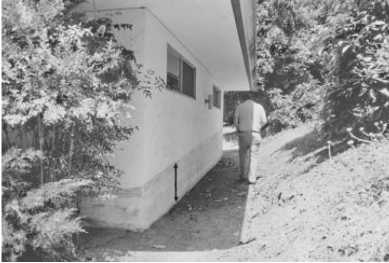
FIGURE 10.47 Photograph of site. Arrows indicate height of the debris flow.
