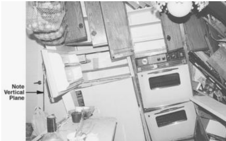
FIGURE 10.6 Damage to kitchen area.
