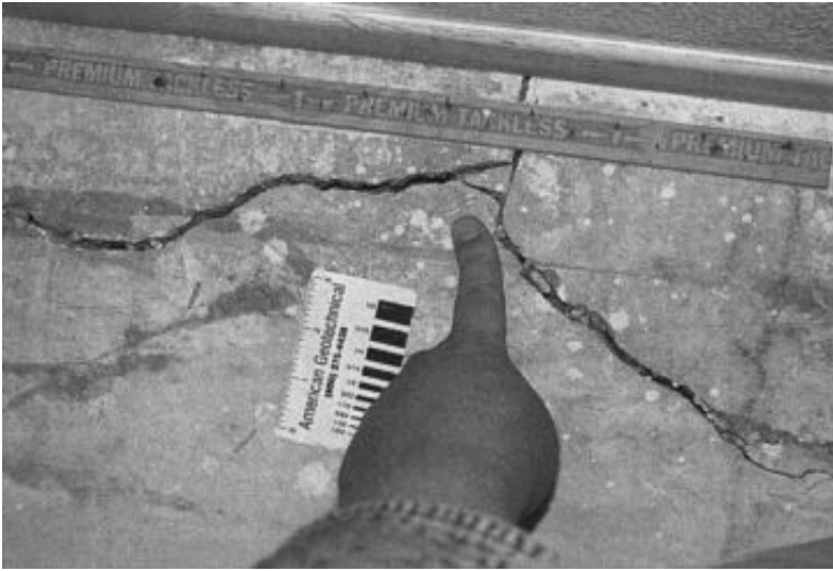
FIGURE 12.11 Excessive shrinkage cracks in a concrete slab-on-grade foundation.
