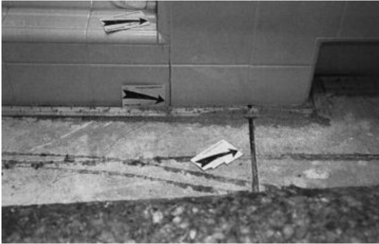
FIGURE 12.16 The opening of a contraction joint (lower arrow) has resulted in the cracking of shower tiles (upper arrow) that span the contraction joint.
