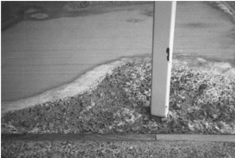
FIGURE 12.4 Concrete patio deterioration, Mojave Desert (note the salt deposits and deterioration of the concrete surface).
