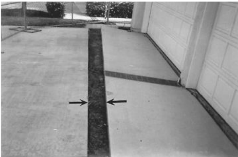
FIGURE 10.38 Laguna Niguel landslide: head of the landslide showing lateral movement of the entire house. (Note: The distance between the arrows indicates the amount of lateral movement.)
