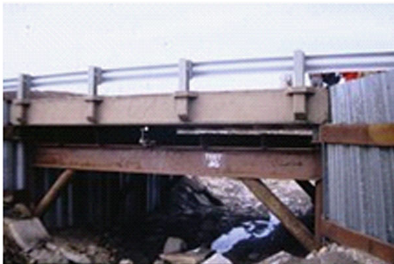
Fig. 16.1 Kansas Structural Composite Inc. No-Name Creek Bridge. Note: Steel structure under bridge is for bridge deflection measurement equipment
