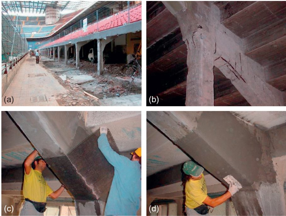
Figure 17.1 (a) Existing RC frame supporting the tier of seats; (b) typical damage found in RC beams; (c) application of a U-shaped TRM jacket for shear strengthening of the beam; and (d) strengthened beam at the end. Kind permission of Ruredil SPA.
