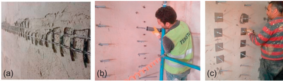
Figure 17.20 (a–c) Strengthening of a masonry wall in the historical building. Kind permission of Fyfe Europe SA.
