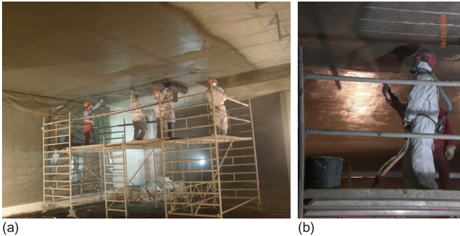
Figure 12.11 Strengthening of the ceilings of a business building in Prague, Czech Republic. (a) Overview (TORKRET GmbH) and (b) spraying of the mortar (TORKRET GmbH).
