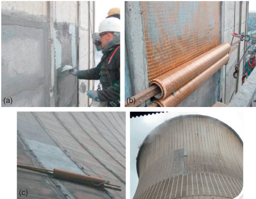
Figure 17.9 (a) Screeding of the inorganic matrix on the tower shells; (b) application of two layers of PBO textile reinforcement; and (c) overview of the strengthening application. Kind permission of Ruredil SPA.
