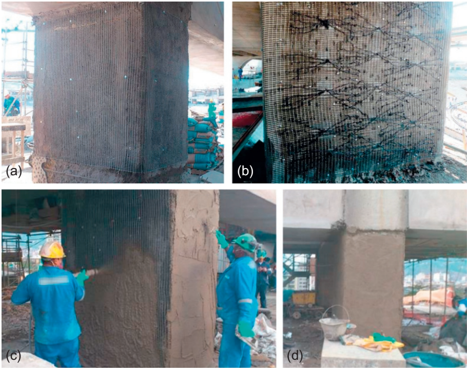
Figure 17.11 (a) Fastening of the carbon textile reinforcement; (b) FRP anchors in wall-like columns; (c) a building worker is spraying shotcrete on the fastened carbon reinforcement; and (d) strengthened column at the end.
