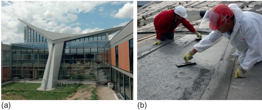
Figure 12.9 The hyper-shell structure in Schweinfurt. (a) Overview (TORKRET GmbH) and (b) application of TRC through spraying with final laminating process (TORKRET GmbH).
