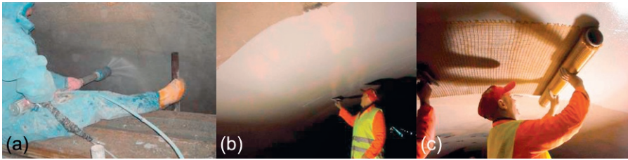
Figure 17.6 (a) Surface preparation by hydrojetting; (b) application of the inorganic matrix; and (c) application of the PBO textile reinforcement.
