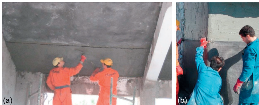
Figure 17.4 Strengthening of (a) concrete slabs and (b) stone masonry walls in a mixed concrete–masonry school building. Kind permission of Triantafillou (2007) .
