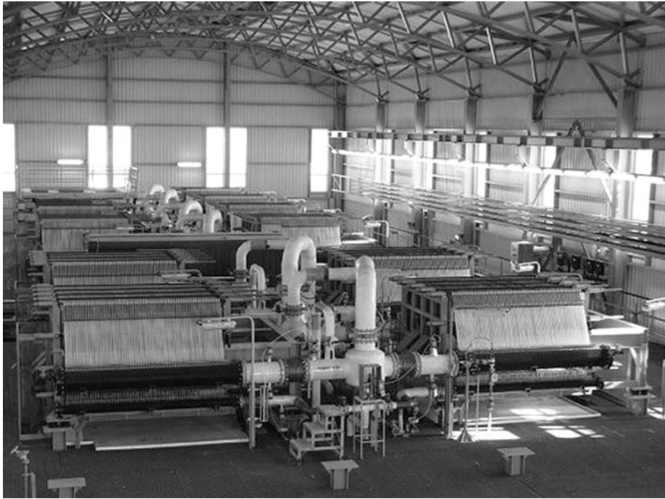
Fig. 26.6 Membrane-cell installation at BorsodChem Zrt., Kazinbarcika, Hungary (Courtesy of Chlorine Engineers Corporation, Ltd.)
