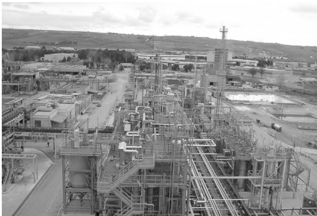
Fig. 1.2 Crompton's silane unit, Termoli, Italy. Courtesy Crompton Corporation
