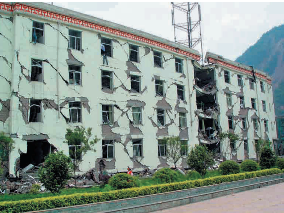
Figure 1.26 Yingxiu middle school, Yingxiu Town in Wenchuan County. The lowest storey collapsed completely and walls show many X shape cracks.
