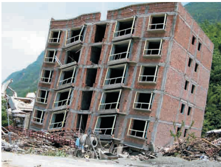
Figure 1.22 Beichuan County, located on the central part of Longmenshan fault zone, suffered devastating destruction. This five-storey brick masonry residential building in Beichuan suffered severe damage, did not collapse, and had to be removed.
