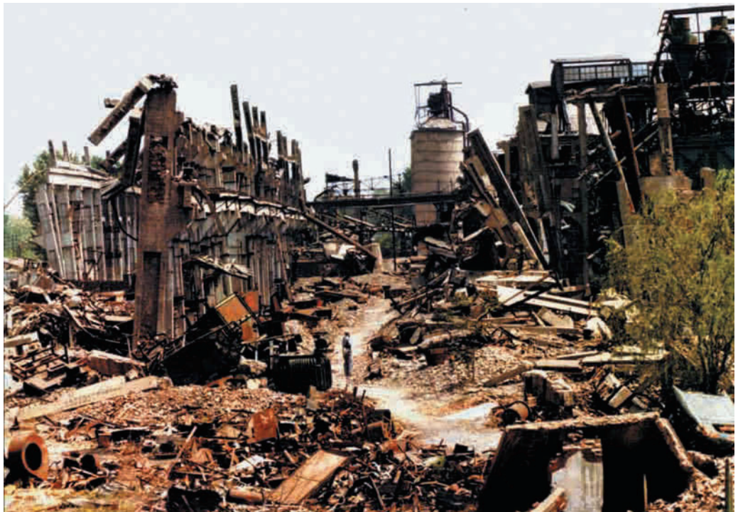
Figure 3.18 Tangshan earthquake ( M7.8 ) of 1976 destroyed a major industrial city Tangshan in a moment and killed 240,000 people. Heavy damage sustained by a part of Tangshan City located within the intensity X zone.
