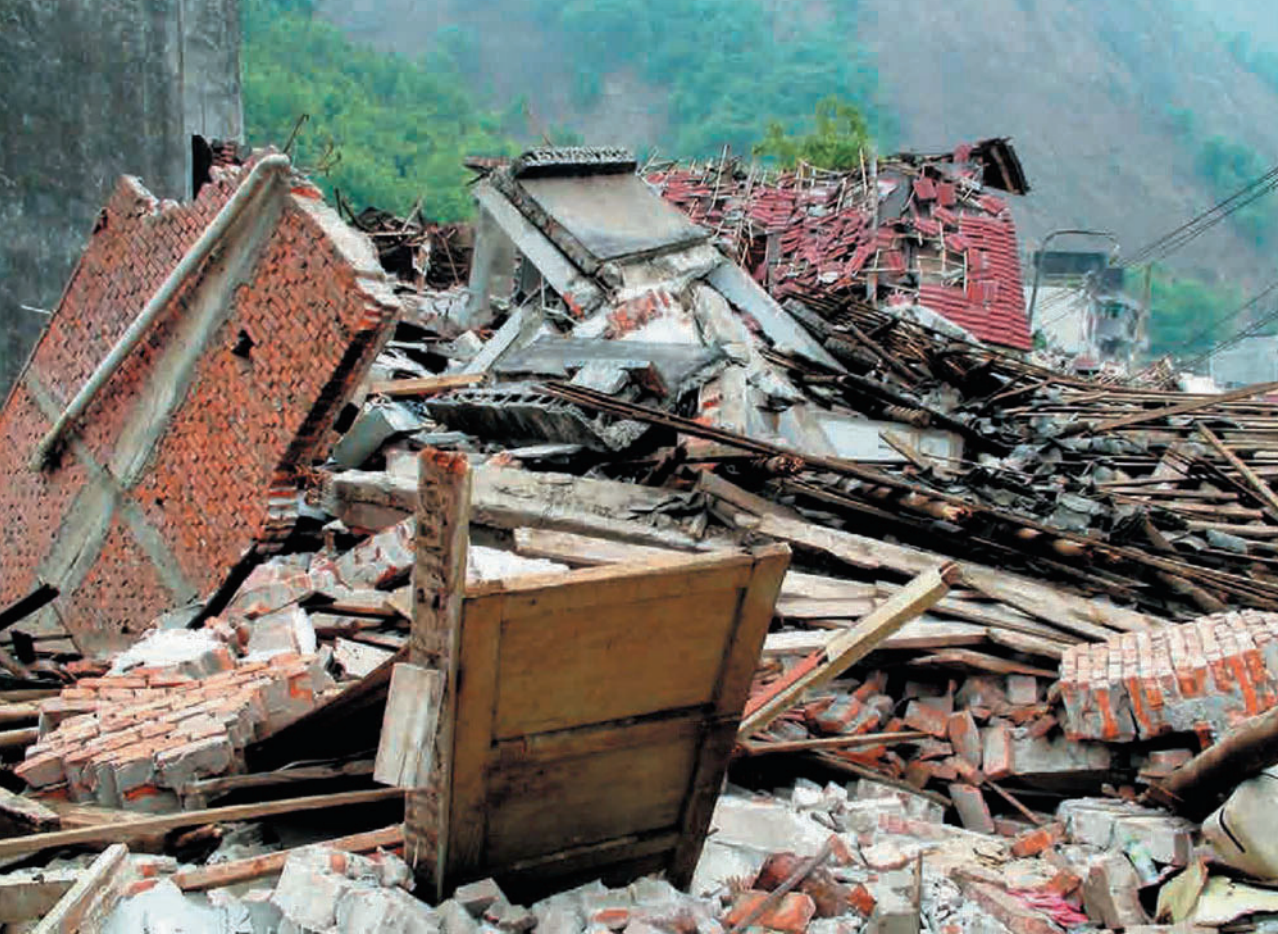
Figure 1.9 Collapsed brick masonry buildings in Beichuan County. (intensity XI)
