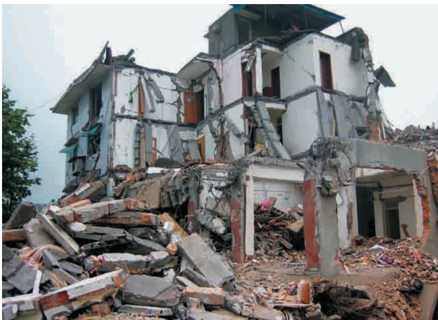
Figure 1.10 Three-storey buildings with a frame structure in the lower part and brick masonry structure in the upper part, were severely damaged. Hanwang Village of Mianzhu City. (intensity X)
