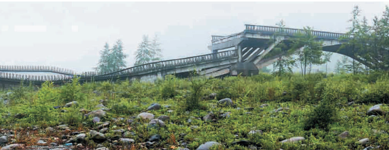
Figure 1.35 Under strong shaking in rural areas, many of the old stone bridges suffered serious damage. Collapse of stone arch bridges in (a) Beichuan (Chenjiaba), (b) Bailu Village, Pengzhou.
