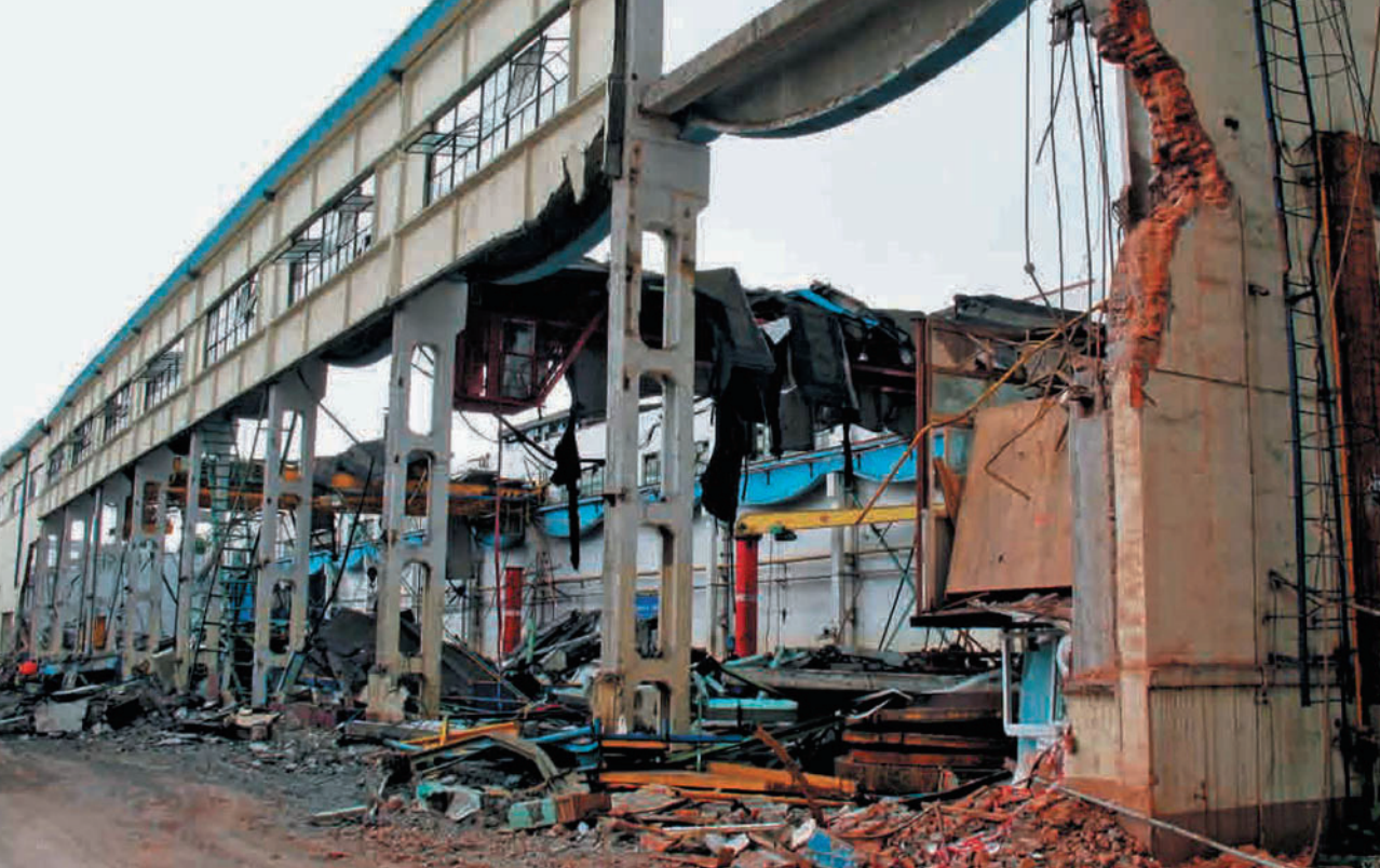
Figure 1.27 Damage to factory buildings at Dongfang Steam Turbine Works (DFST) in Mianzhu City is representative. Most buildings used traditional bent columns. The precast truss, and ribbed roof slab collapsed entirely, causing serious losses of life and facilities. Fortunately, seven similar buildings survived the earthquake thanks to the lightweight colored sandwich steel plate or corrugated steel replacing the precast ribbed roof slab a few years ago. Factory buildings with steel trusses remained basically intact thanks to their satisfactory bracing system, despite using a heavy precast ribbed roof slab. Factory buildings using a portal frame withstood the earthquake well.
