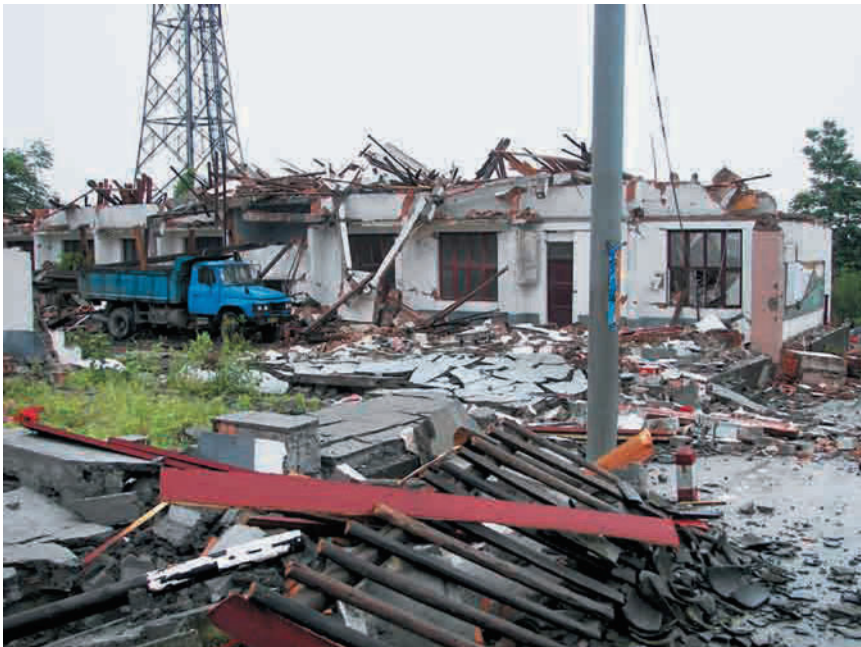
Figure 1.42 Destruction of mobile communication station in Wudu, Gansu Province, 450 km far from epicenter.
