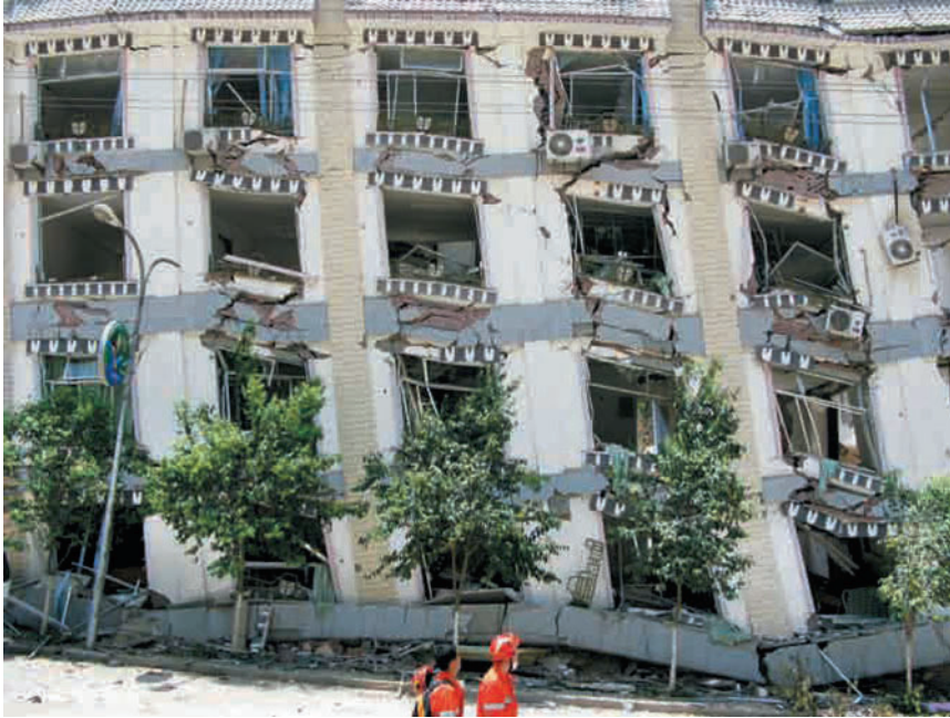
Figure 1.24 Beichuan middle school: five-storey reinforced concrete frame structure. Entire collapse of ground floor, and upper 4 storeys damaged severely. Assigned for demolition.
