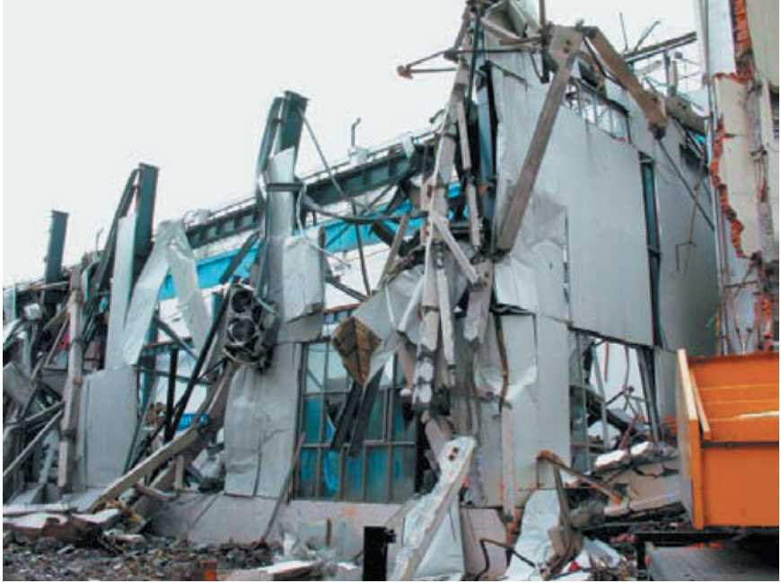
Figure 1.11 Damage to a building of Dongfang Steam Turbine Works (DFSTW) in Mianzhu City. Most of these buildings, built of bent columns, PC trusses, and precast ribbed roof slabs, collapsed entirely, causing serious loss of life and facilities. (intensity X)
