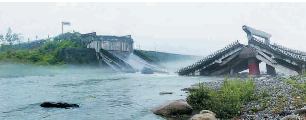
Figure 1.34 Pengzhou, Xiaoyudong bridge, bridge collapse of two cross (courtesy of Lu Ming).
