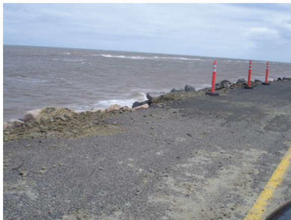
Fig. 2.16 Damages on road 113 on the island of Miscou, New Brunswick, Canada. Source S. Weissenberger, 2012
