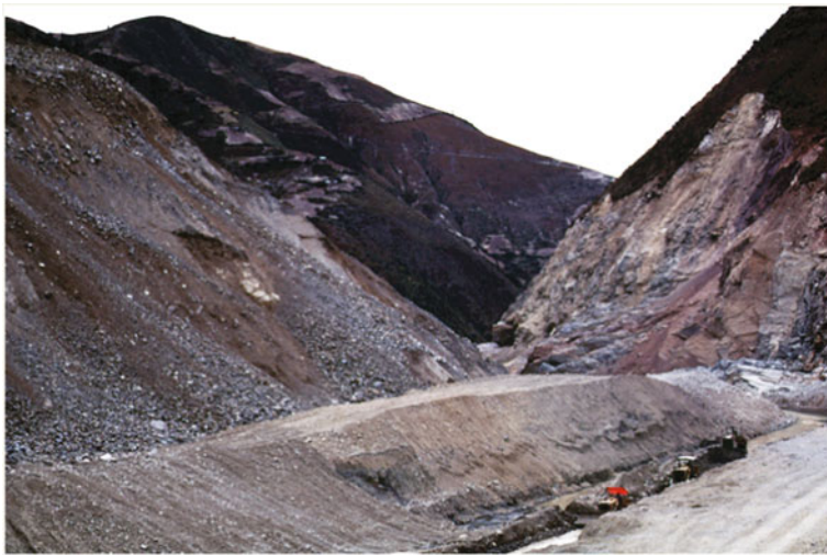
Fig. 3.16 Excavation of a new channel in the landslide mass after the May 1st, 1993 overflow. The unstable left slope that required a stabilizing scheme can be observed
