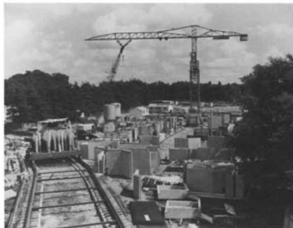
Figure 4.1 University of East Anglia: battery casting on site with lightweight coarse and fines concrete, circa 1965.
