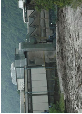
Fig. 7.2. Damage to an industrial site in Val Chisone, Italy, 2008
