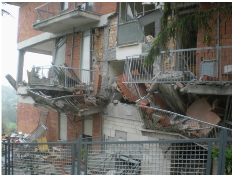
Fig. 13.7 L'Aquila city: reinforced concrete (RC) frame building that has suffered mid-floor compression
