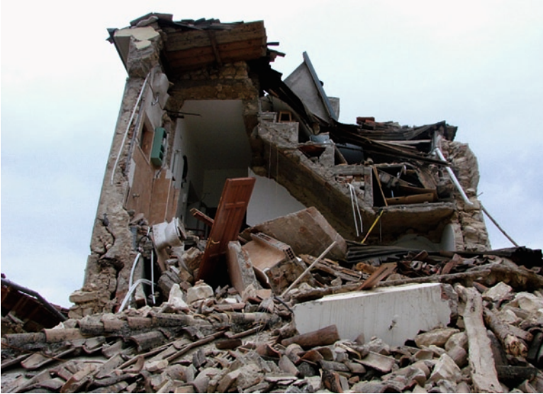
Fig. 13.6 Partially collapsed unreinforced brick masonry building (URM) at Onna, L'Aquila municipality
