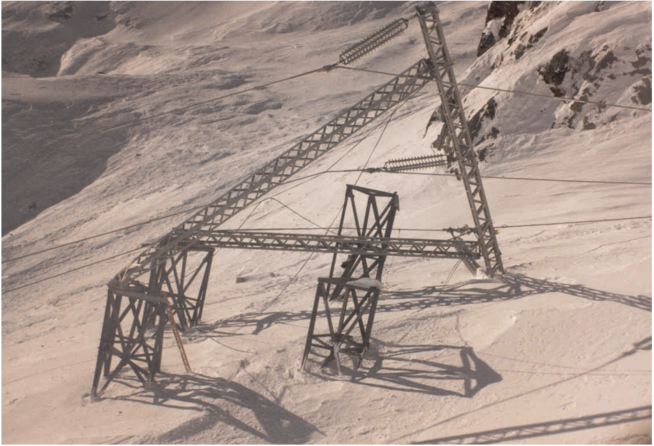
Figure 7.7 The fallen hinged tower
