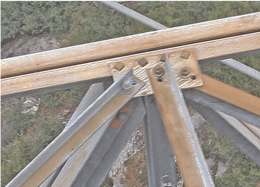
Figure 7.10 Missing bolts in 'Tower Bridge'
