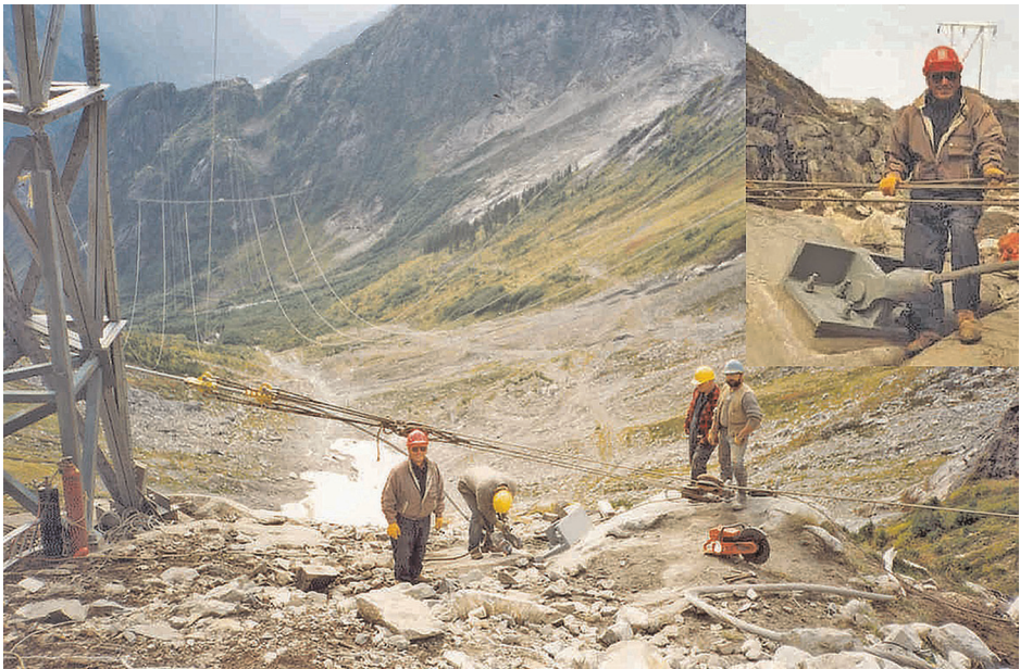
Figure 7.9 Remaking the failed temporary anchorage. (Inset) Adam Charneski
