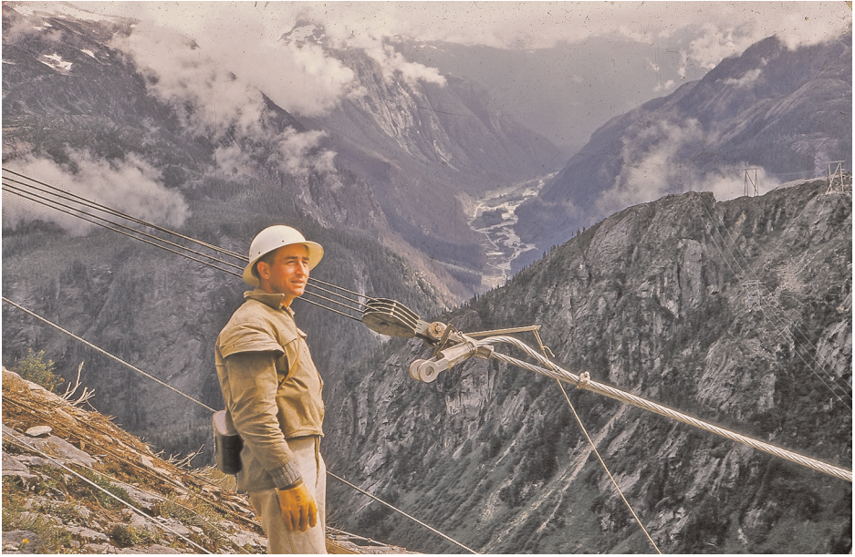
Figure 6.1 Brian White, aged 32, standing at his catenary site while its cable is pulled to the anchorage. The Kemano River valley is in the background, 1000 m below. (Courtesy of H. Brian White)
