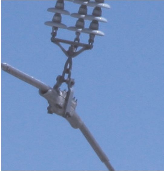
Figure 4.15 A three-bundle suspension string yoke. (Courtesy of Peter Catchpole)
