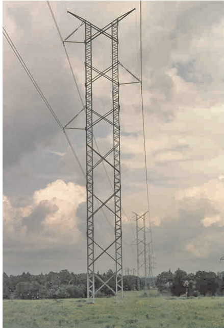
Figure 4.6 A frighteningly tall H frame structure. (Courtesy of Peter Catchpole)
