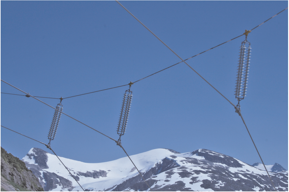
Figure 6.7 The KitiKat supporting about 25 tonnes of conductors
