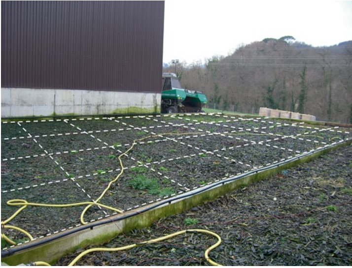
Fig. 2.2 Image of fictitious partition of a biofilter surface to undertake the measurement of air velocity and gaseous emissions
