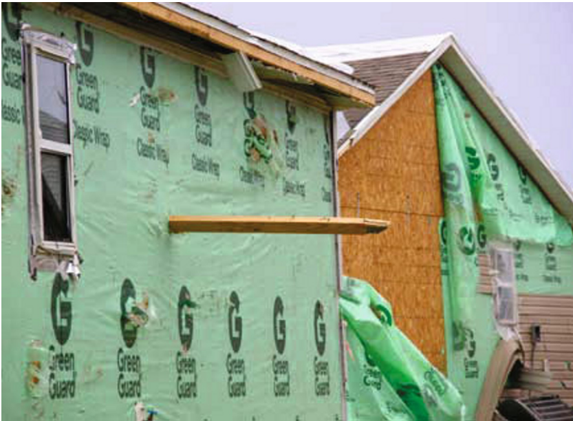
February 2, 2007: Missile impacts a home on Norris Way, in the Village of Mallory Square, The Villages, Florida. EF-3 tornadic winds producing degrees of damage (DOD) of 3-8.
