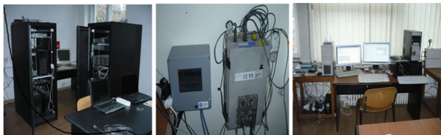
Fig. 17.1 Views of the seismic data recording, processing and storage equipment installed at INCERC
