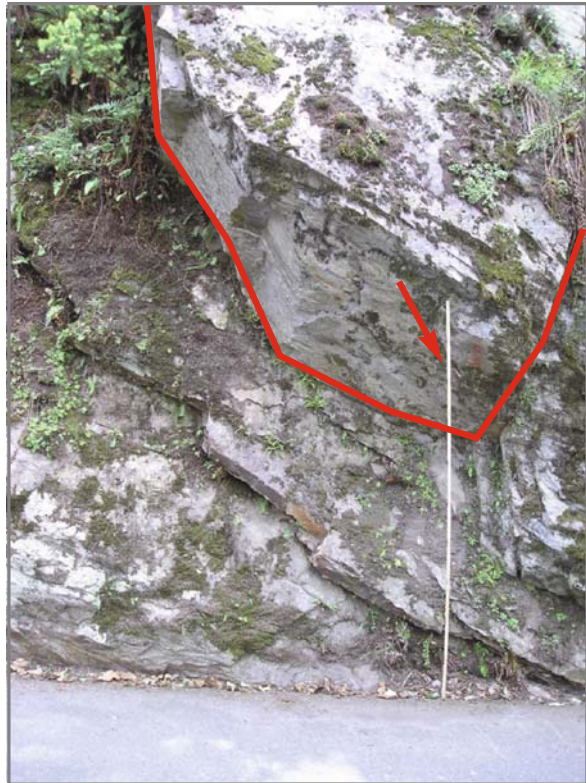
Fig. 6.31 Discontinuity families that divide the rock in blocks and possible direction of the movement
