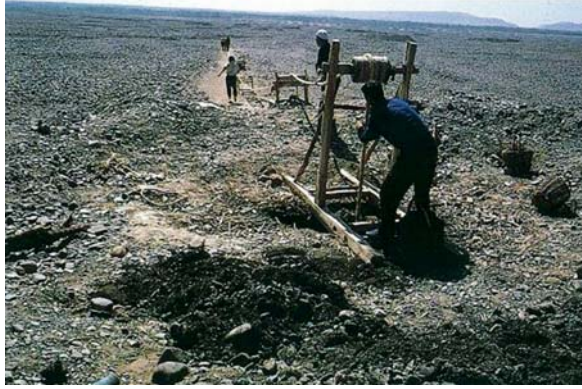
Fig. 9.5 Cleaning an underground tunnel of a karez in Turpan. (Source: the author)
