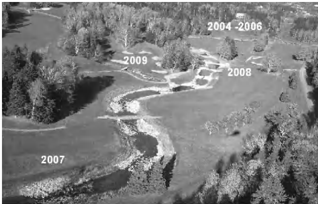
Figure 25. Pool and riffle profile constructed between 2004 and 2009 by Parks Canada staff in the formerly channelized reach of Dickson Brook as it flows through Fundy National Park golf course, New Brunswick. Riparian vegetation has been planted in nonplay areas. Cover boulders and tree wads are added to the reaches in fairways. Photo by J. Watts.
