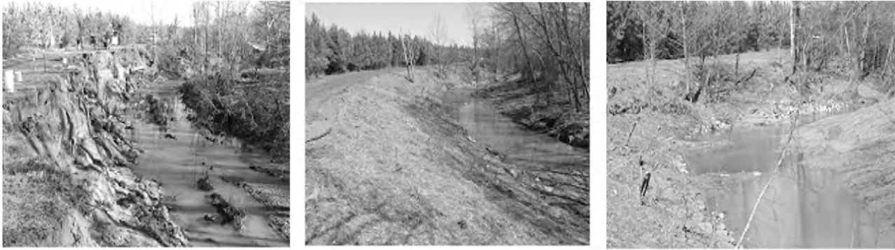
Figure 3. View of the bendway looking upstream (left) from January 2006 and immediately following construction in March 2007. (middle) Note edge of constructed rock riffle in lower right and (right) stone-toe protection with three bendway weirs. From the work of Simon et al. [2008], reprinted with permission from ASCE.
