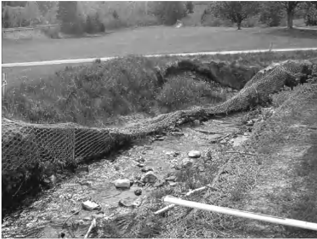
Figure 24. A typical gabion basket and lined channel failure in Dickson Brook 10 years after installation.
