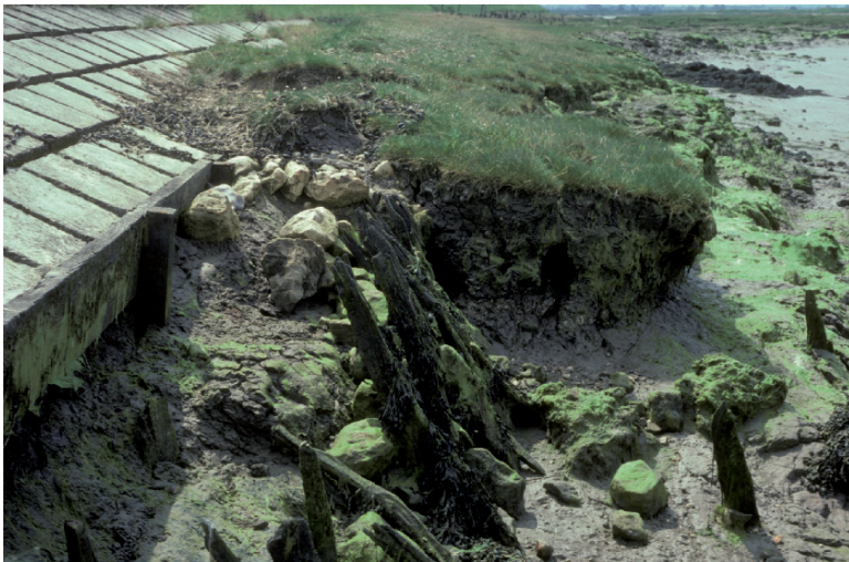
Figure 42 Eroding saltmarsh undermining a sea wall, Essex
