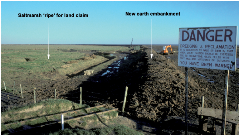
Figure 19 Erection of an earthen embankment, southwest shore of the Wash in the late 1970s
