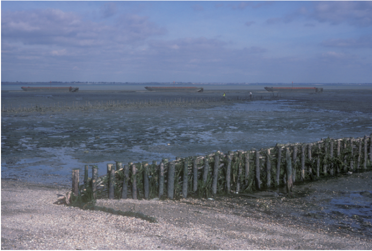
Figure 47 Construction of shore-linking groynes 1989, Sales Point, Dengie, Essex, UK. In the distance, Thames barges sunken in situ
