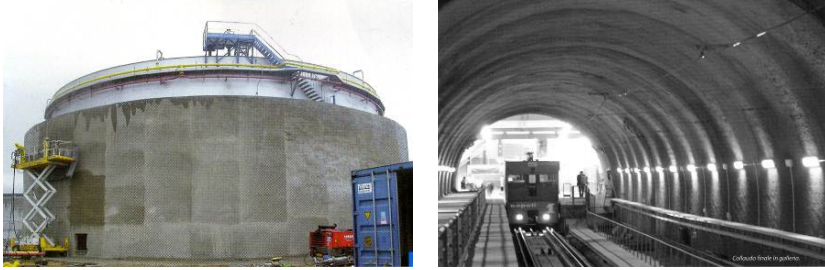
Fig. 1. Structural use of shotcrete (left) in a cylindrical shield for the protection of an oil tank (France, Atlantic Coast); and use of sprayed mortar (right) for water-proofing the lining of an urban tunnel (Italy, Naples), both from Realtà Mapei, V. 96, N.9, 2009.
