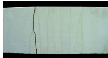
Fig. 4. Multiple cracking on the tensile face after the flexural test
