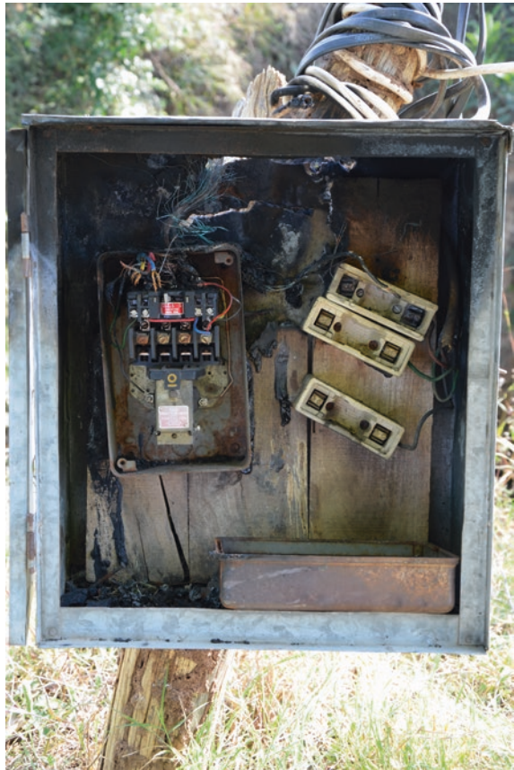
Fig. 7.10 Burned out starter panel. Source Malte Müller
